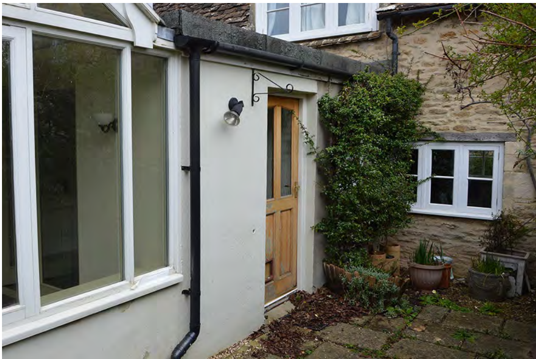
Plate 12 Kitchen extension (centre right with greenery) and lobby extension (centre with door)
