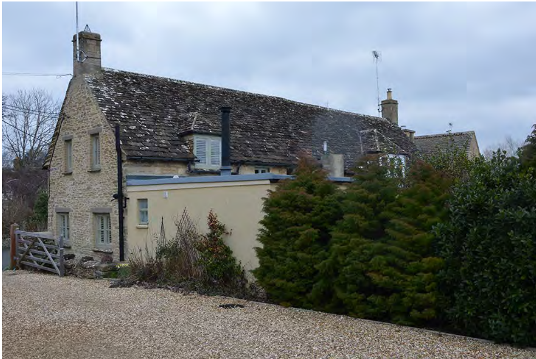
Plate 17 Quoice Cottage north west elevation before and after chimney removal (left photo provided by Poole Phillips)
