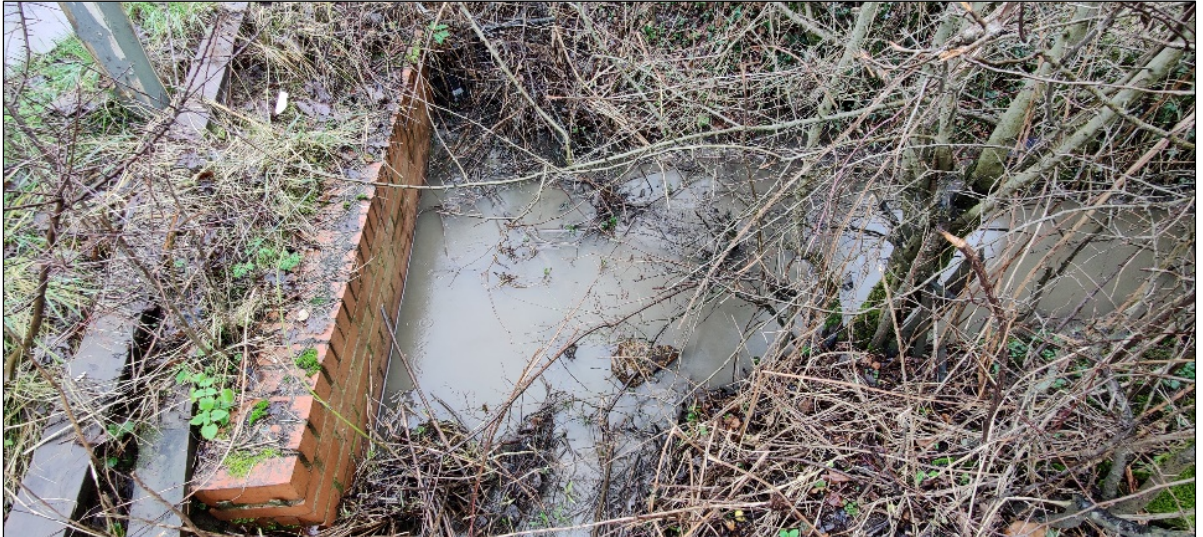
Figure 10 - Blocked Culvert at Vicarage
