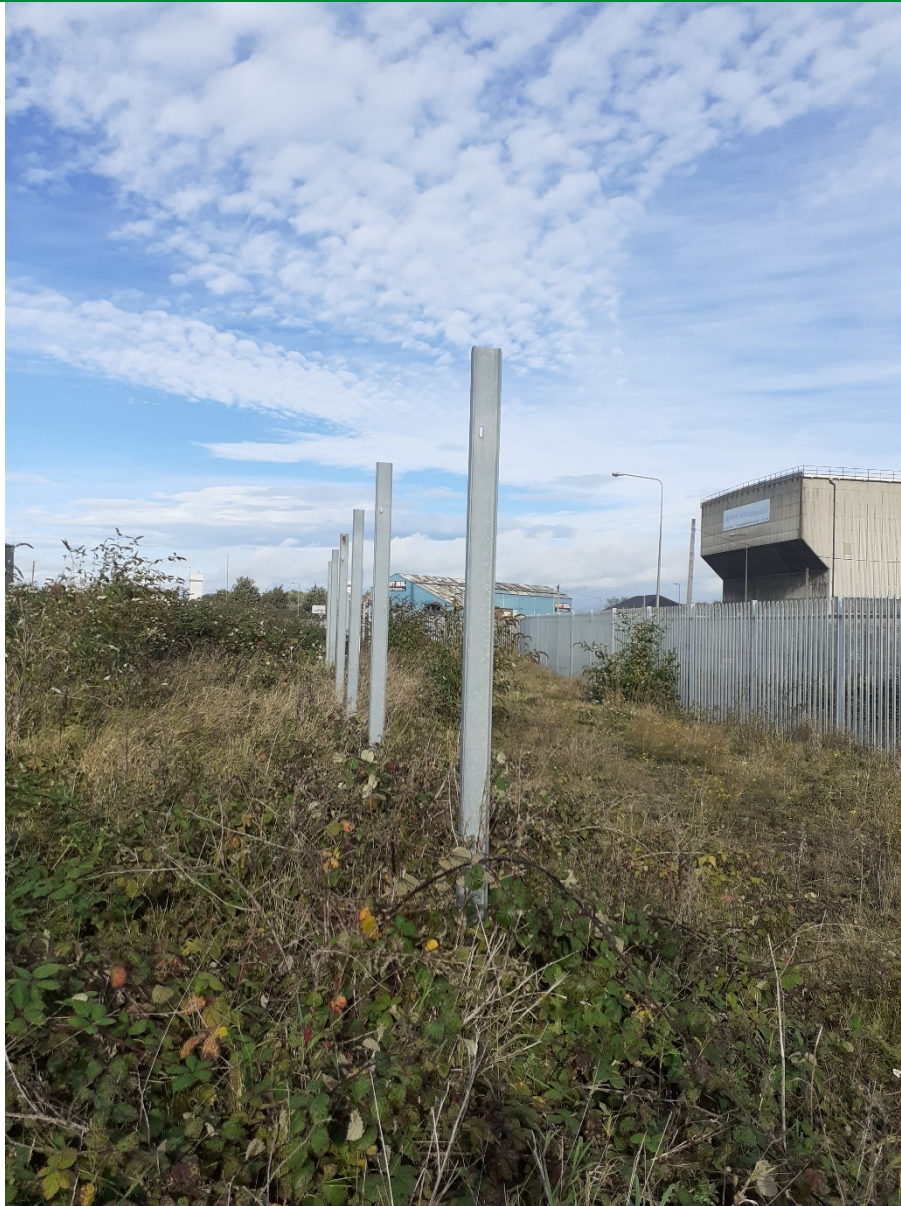
PLATE 7 – FENCE ALONG EASTERN BOUNDARY, NOTE PARTIALLY BUILT FENCE
