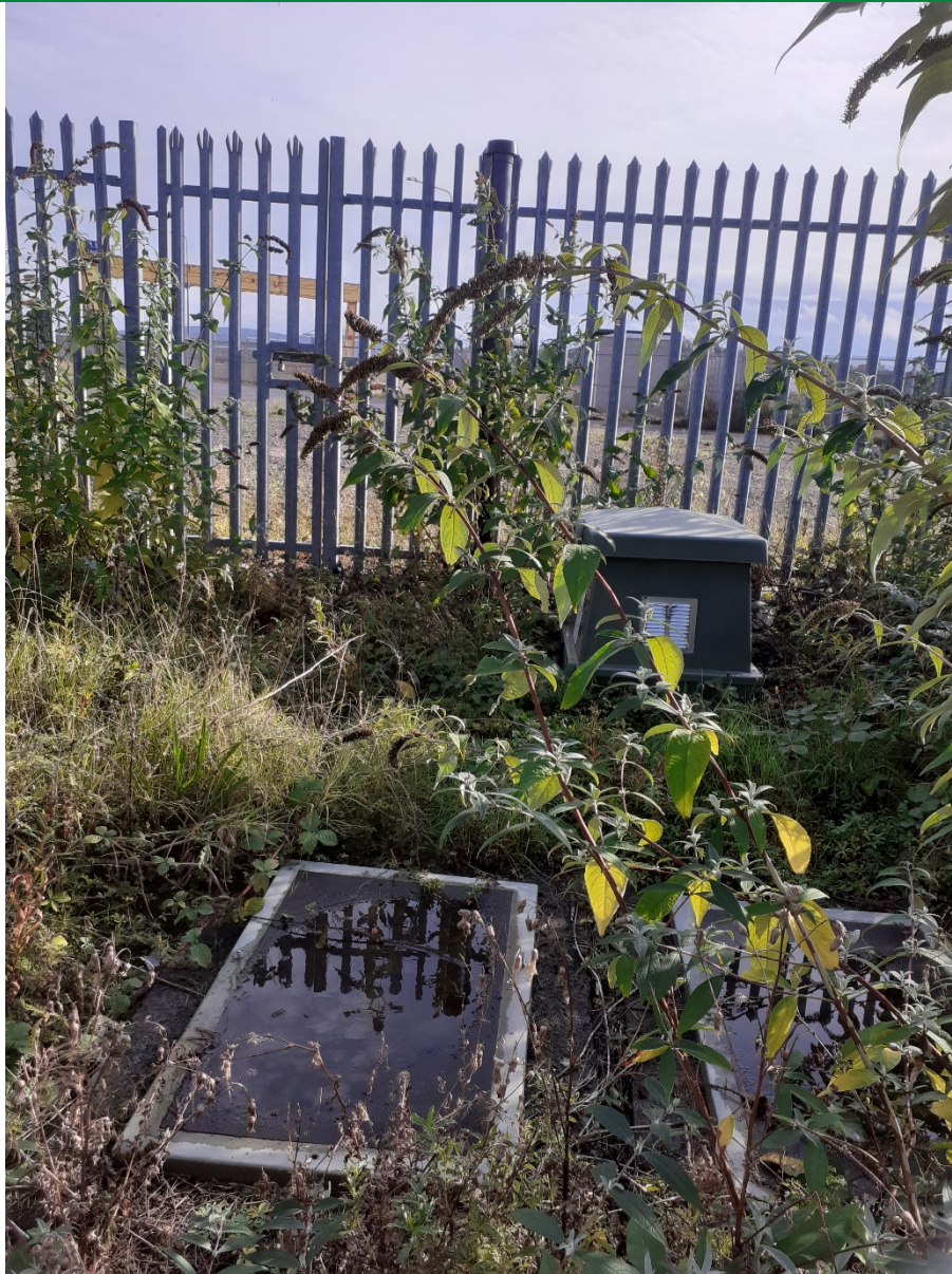
PLATE 9 – FENCED OFF SERVICE – ANECTDOTAL EVIDENCE SUGGESTS THAT THIS IS A SWITCH PUMP ASSOCIATED WITH NEIGHBOURING SHIP YARD
