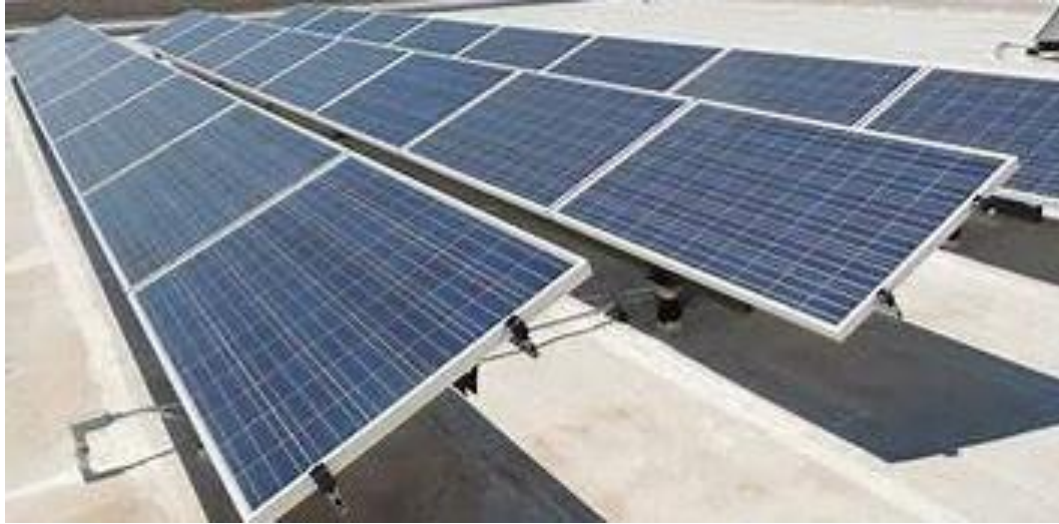
Solar Photovoltaic Panels
