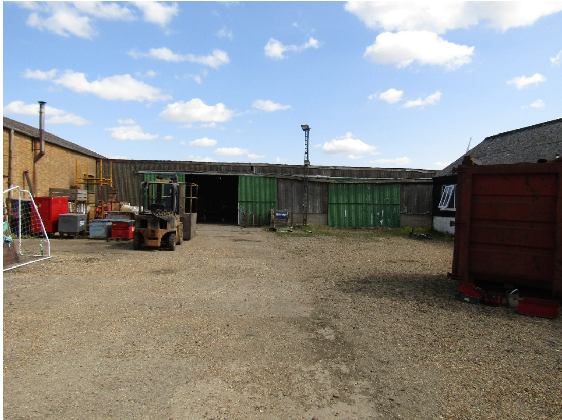
Photo 1 , looking north towards the southern aspect of the barn with large sliding doors.
