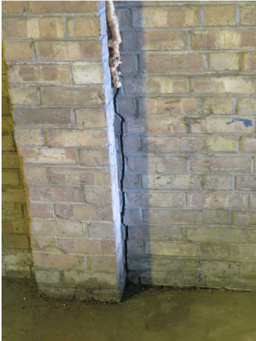
PHOTO No. 9 – VERTICAL CRACK ADJACENT TO PIER FILLED WITH FOAM FILLER
