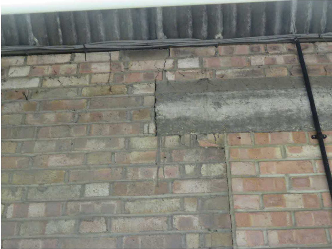
PHOTO No. 7 – VERTICAL CRACK AT FILLED IN DOOR OPENING
