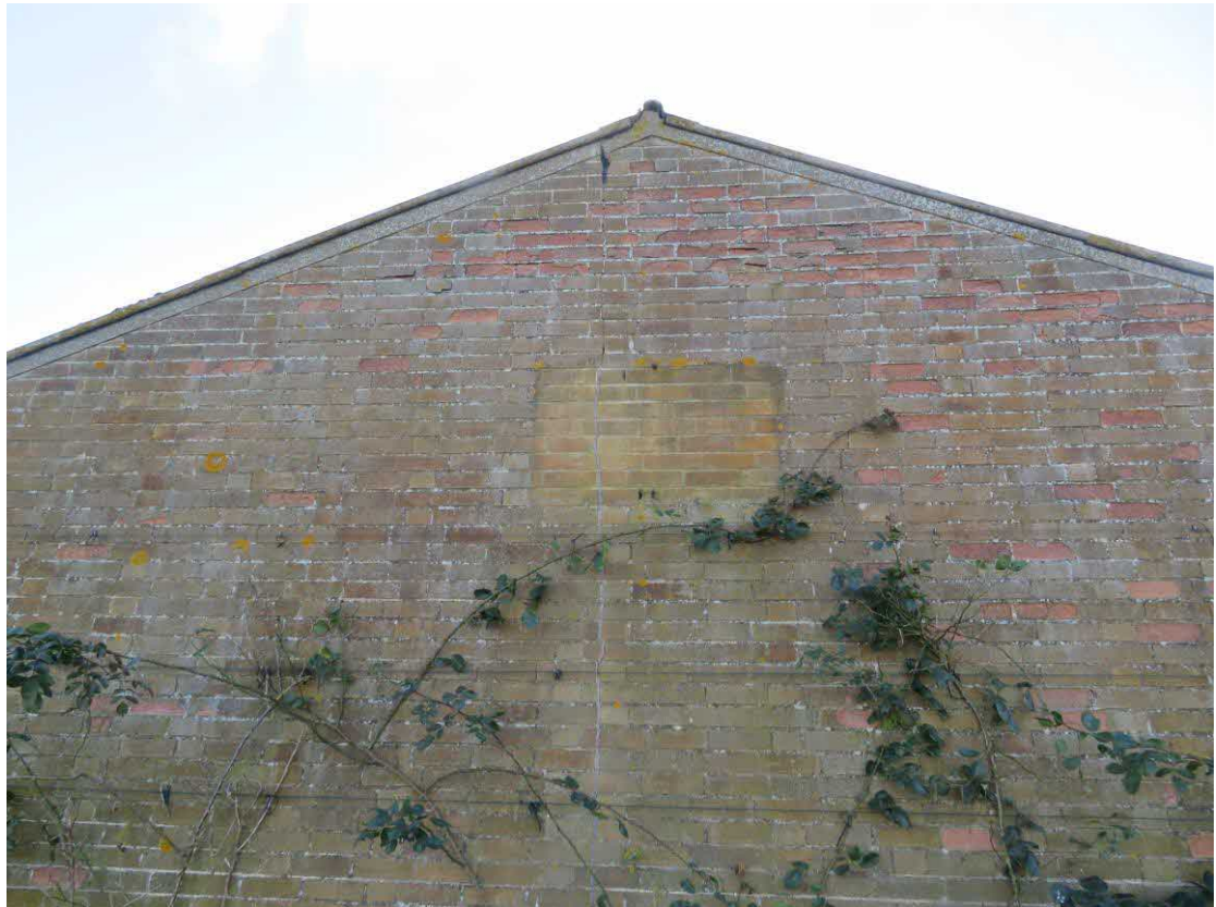
PHOTO No. 4 – VERTICAL CRACK IN NORTH GABLE
