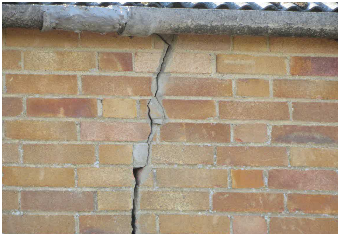
PHOTO No. 6 – VERTICAL CRACK ON EAST ELEVATION
