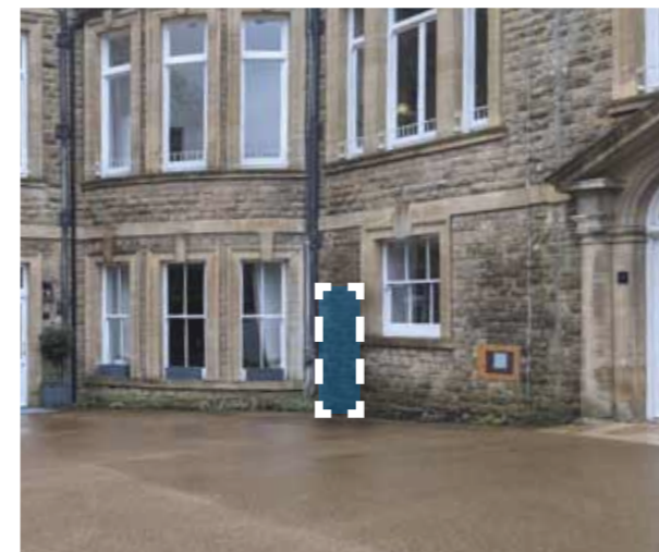
Apartment 11 - External socket & switch location on facade
