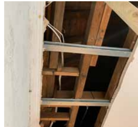
Ceiling void / roof required full review of insulation
