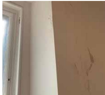
Paint peeling off the walls
