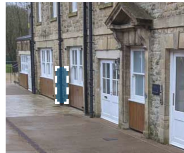
Apartment 10 - External socket & switch location on facade
