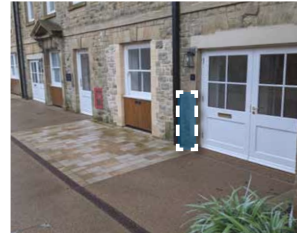
Apartment 09 - External socket & switch location on facade
