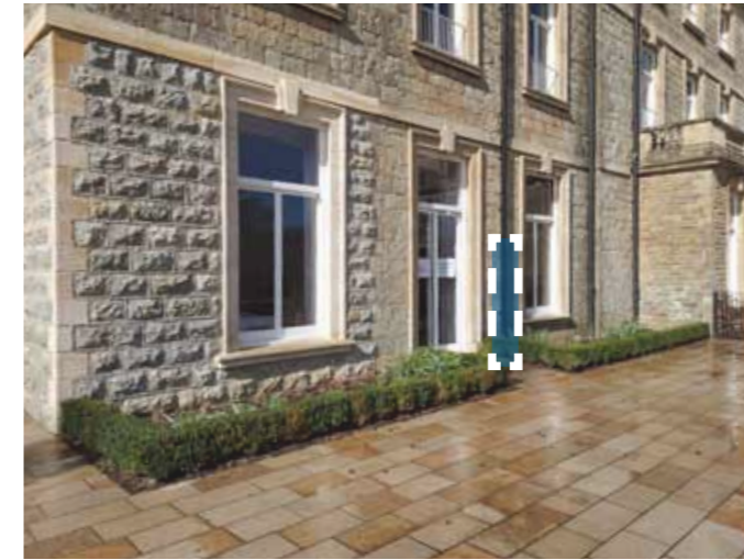
Apartment 14 - External socket & switch location on facade
