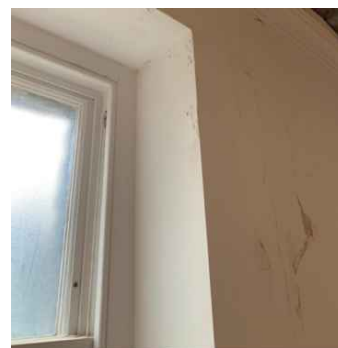
Paint peeling off the walls
