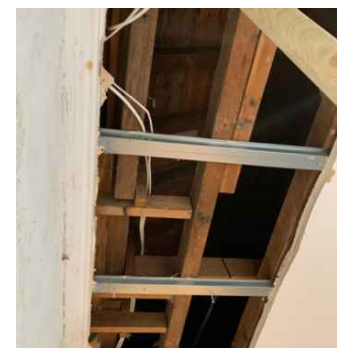
Ceiling void / roof required full review of insulation
