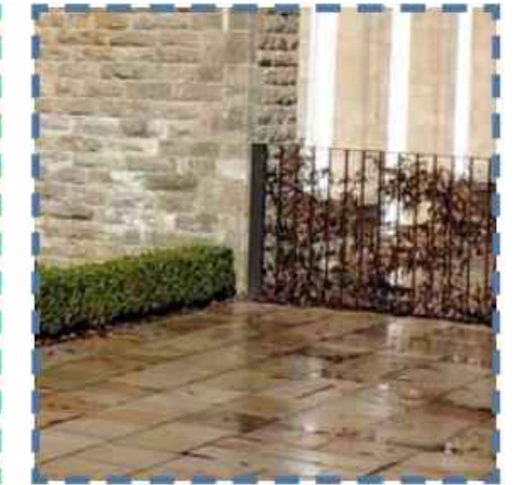
Railing dividing apartments 13, 14, and 15 terraces allow for planting along one side and are not fixed back to the building facade.
