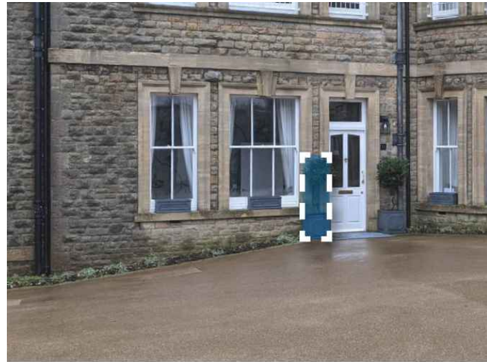
Apartment 12 - External socket & switch location on facade
