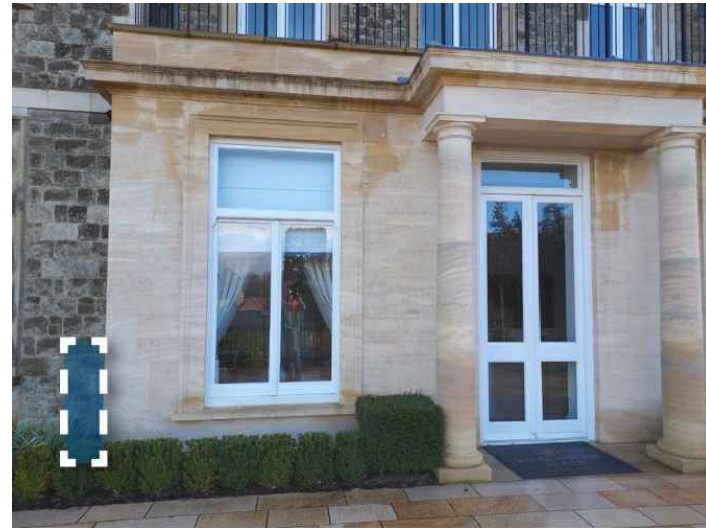
Apartment 13 - External socket & switch location on facade
