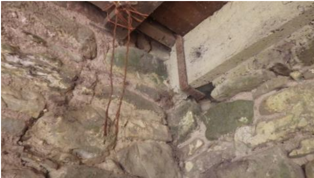
Photo 19: Northern wall with crevice down wall
