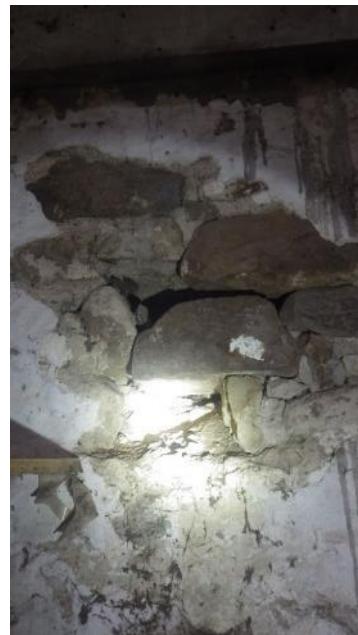
Photo 10: Deep crevice within stonework on eastern aspect of room 1
