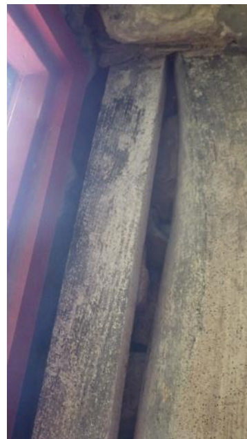
Photo 16: Gaps along door frame providing roosting potential
