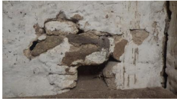
Photo 8: Gaps in stonework in room 1
