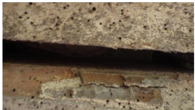
Photo 14: Large gap on door lintel with roosting potential
