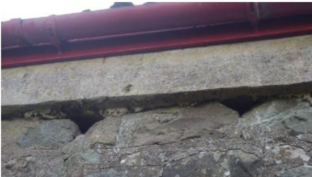
Photo 5: External wall on east aspect with deep gaps on stone wall
