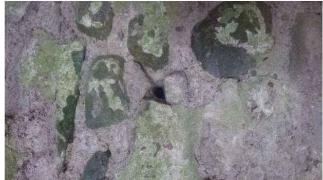
Photo 20: Hole in stone wall along eastern aspect
