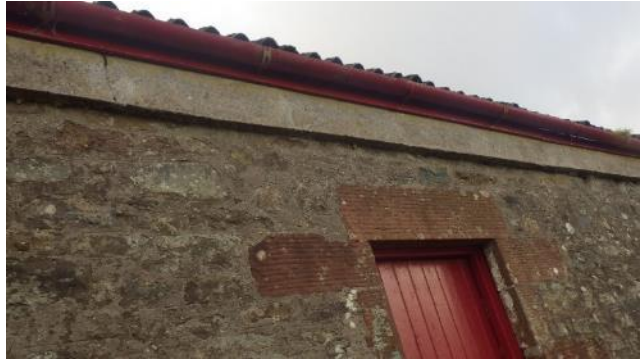
Photo 4: East aspect of steading showing gaps around door frame
