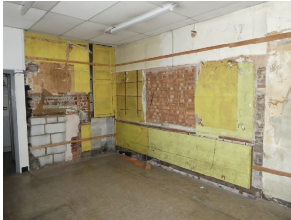
Figure 10: Evidence for a partition, blocked window opening and brick fireplace in the north-east corner of G1
