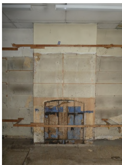
Figure 9: Chimney breast and blocked fireplace on the eastern side of G1
