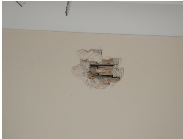
Figure 37: Riven lath and plaster finish on the partition between F8 and F9
