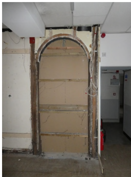
Figure 11: Blocked opening between G1 and the staircase hall to the north (G3)
