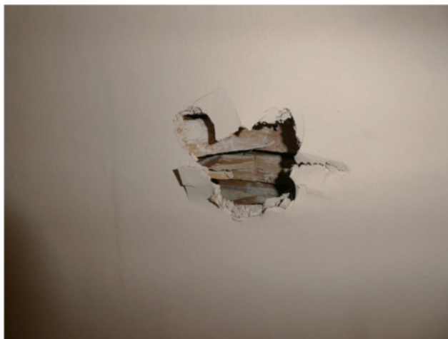
Figure 23: Riven lath and plaster finish associated with the cupboards on the north side of F1
