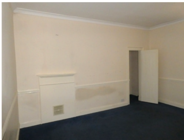
Figure 35: Blocked fireplace and cupboard door in F9
