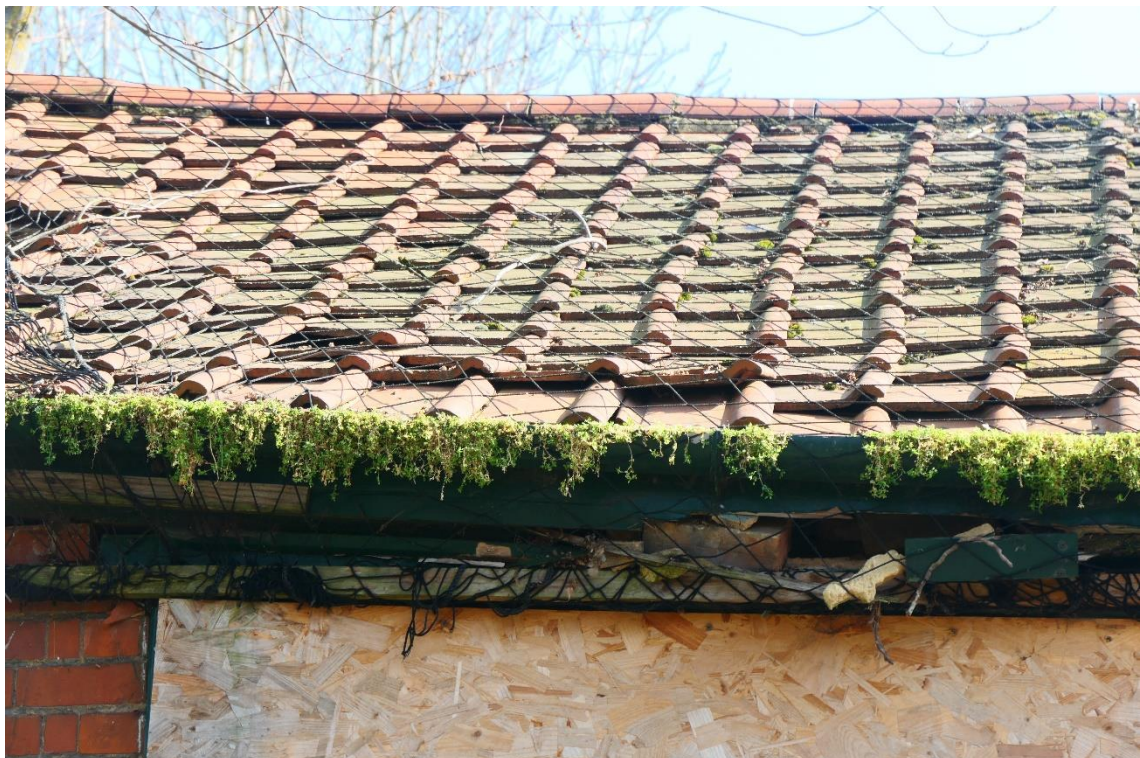
Photo 9 , lifted, damaged and missing roof tiles provide roosting and access opportunities for bats.
