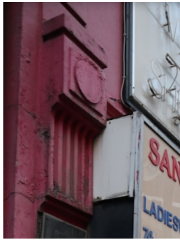
Original console bracket design - left hand of side of unit 74 Middlesex Street to be model for recasting
