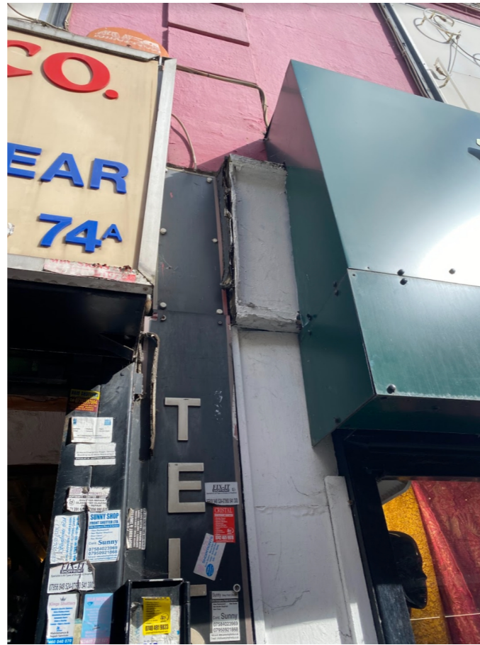
02 Original fascia behind modern box sign
