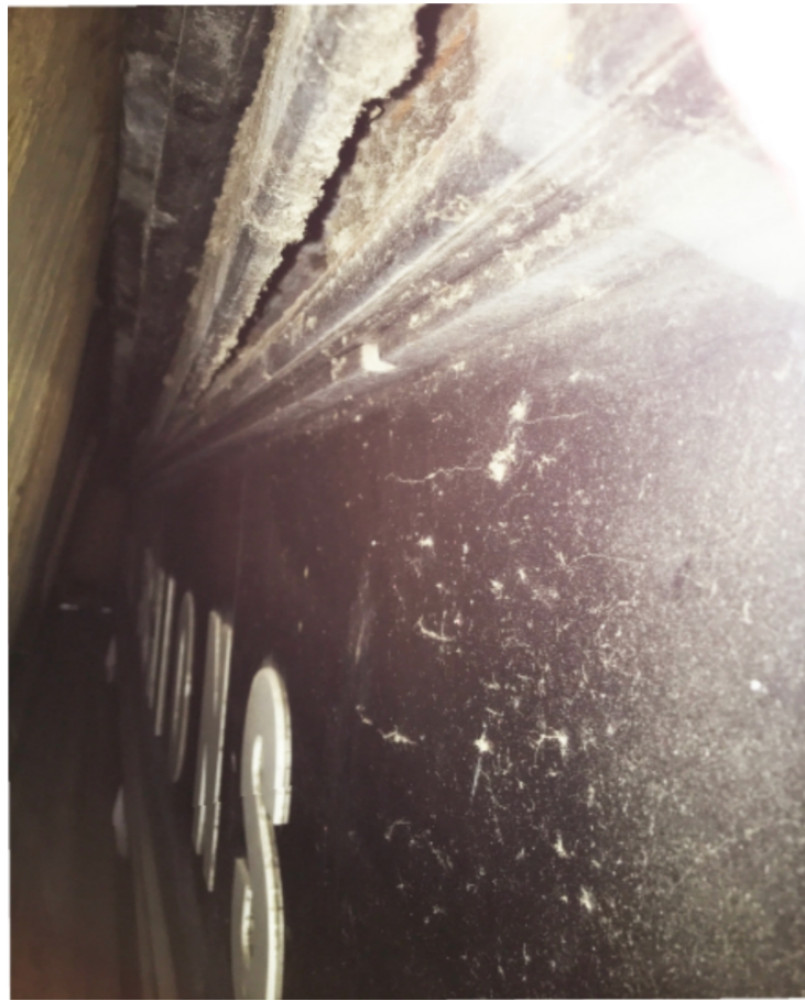
01 Original fascia behind modern box sign
