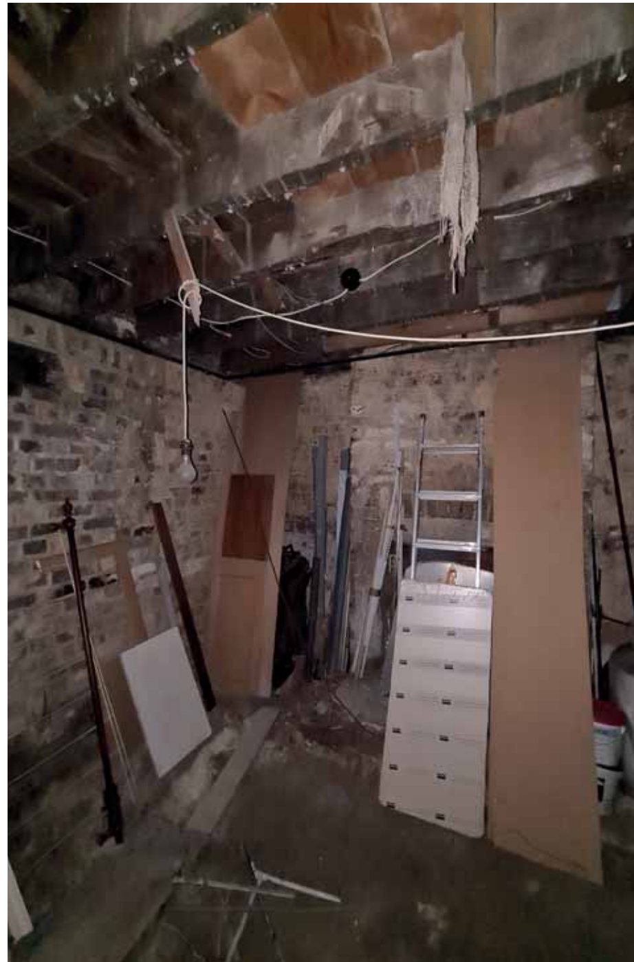
The chimney breasts continue down into the full height cellar, with discernible fireplace openings with brick arches, suggesting prior occupation.
