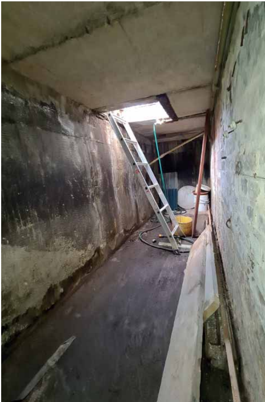
Access to the cellar from the street via a hatch in the concrete slab. This slab is clearly not an original detail, and crashes into what was likely the original window to the cellar. The different colour brick on the right of this photograph shows where the original opening has been infilled.
