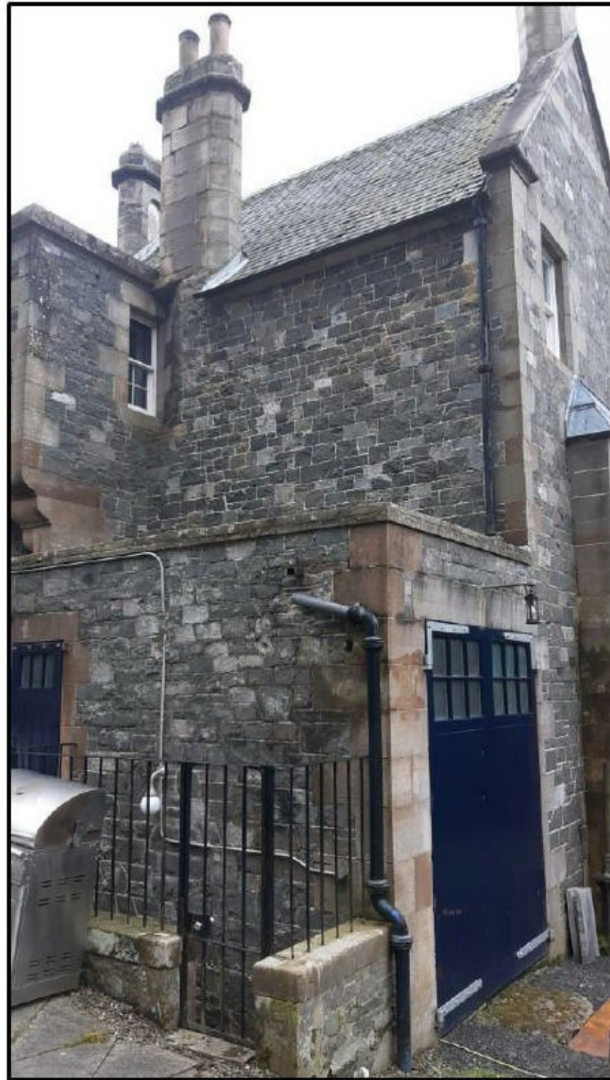
Photo 6: Existing garage and cellar access steps over which a canopy is proposed to be installed. Note existing metal railings and gate.
