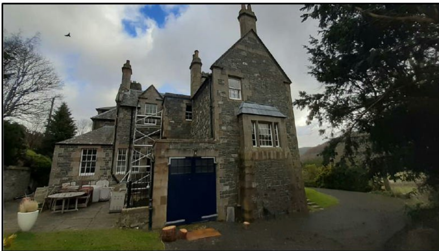
Photo 5: Existing garage and cellar access steps to left (north) over which a canopy is proposed to be installed.
