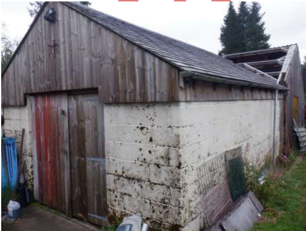
Figure 6 photo 5 view to the east of partially roofed L shaped building (door to staff rest room, stores etc)
