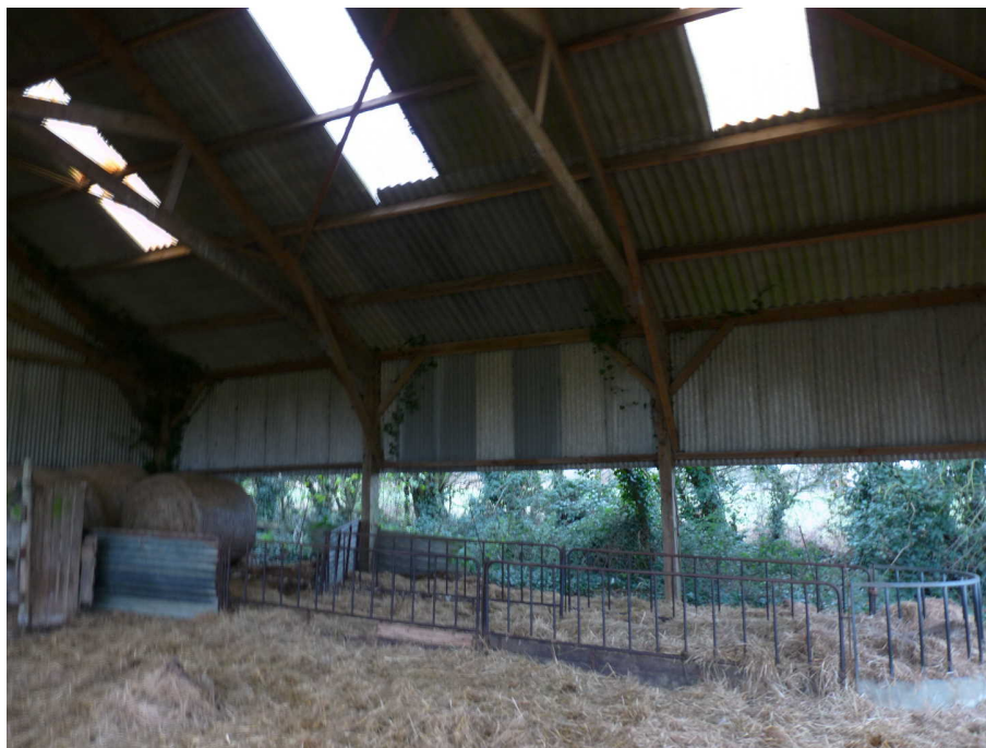
Photo 3: Looking south-west within the barn. Note transparent roof panels, sawn timber beams and ivy growing within the building
