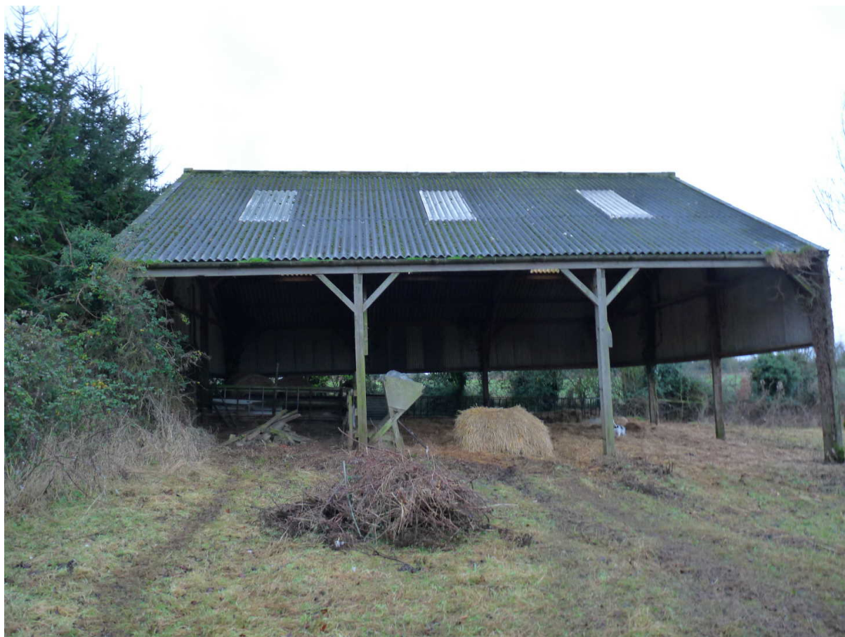
Photo 1: The north-eastern elevation. The other three sides have corrugated asbestos cladding to c. 2m above the ground
