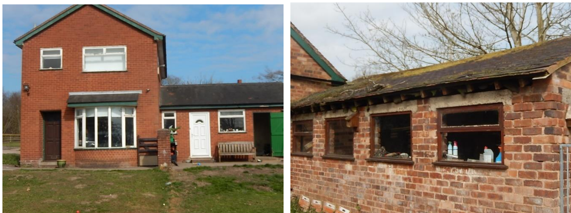
Main dwelling House (left) and kennel building (right) showing gap within eaves as potential entry points
