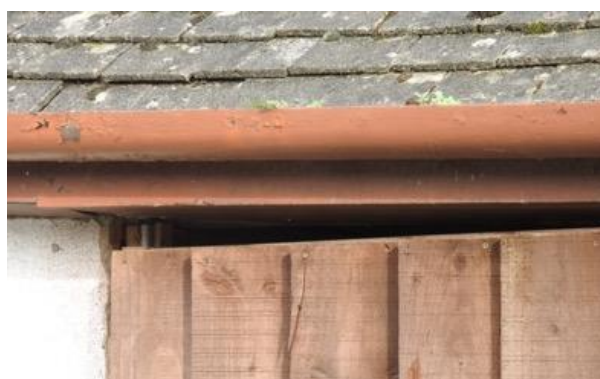
Fig. 28 Door with gaps
