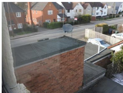
Fig. 20 Tarred felt flat roof to the rear
