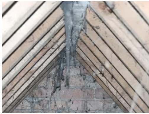
Fig. 17 Cobwebbed ridge and gable end of the perpendicular void
