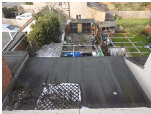
Fig. 10 Tarred felt flat roof to the rear
