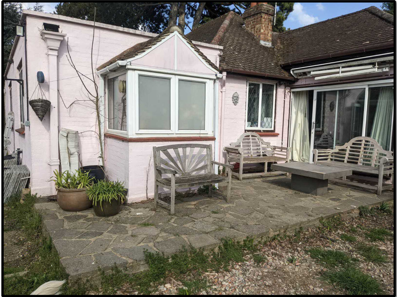
Figure 3 –Photograph of the existing concrete patio. The proposed foundations are aligned to the same footprint.
