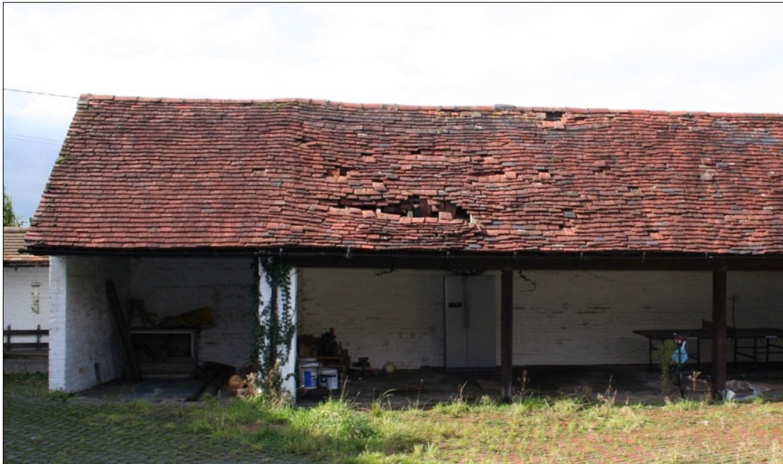
Fig.20 Several outbuildings within the application site are in urgent need of repair.
