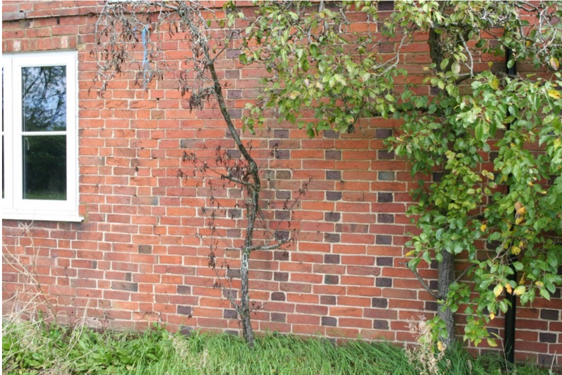
Fig.5 The earliest part of Arbour Tree Farmhouse is identifiable from the use of dark diaper work in the wall and window lintels of the front elevation.
