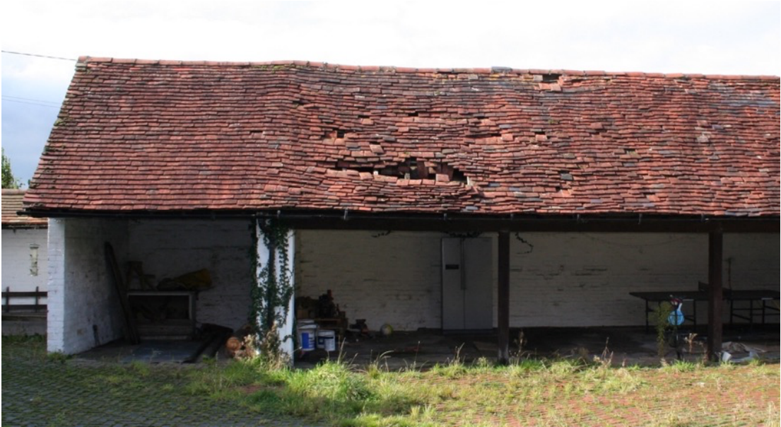
Figure 3 South end of the L-shaped range is in particularly urgent need of repair.
