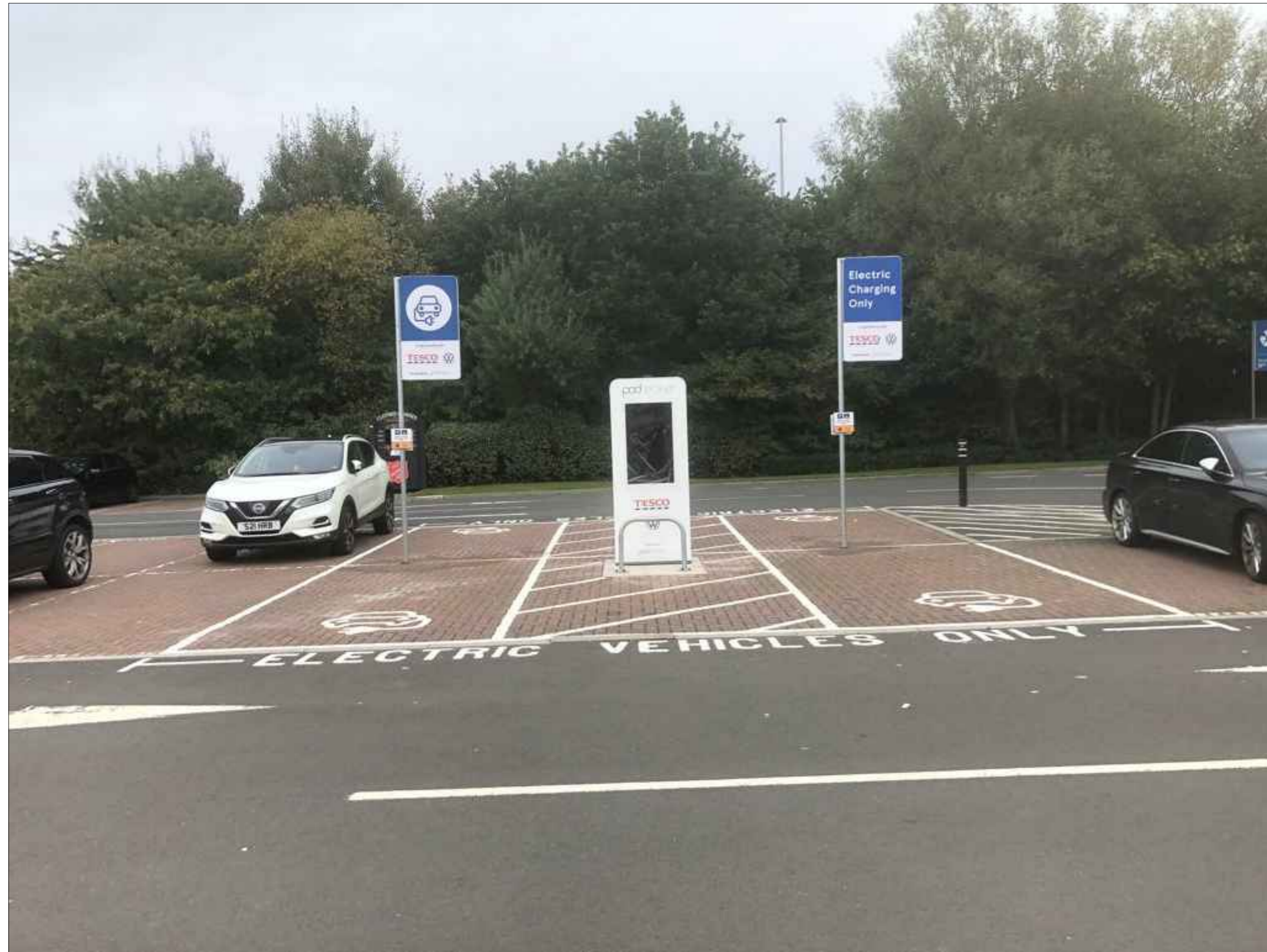
ELECTRIC VEHICLE-CHARGING AREA AT SITE
