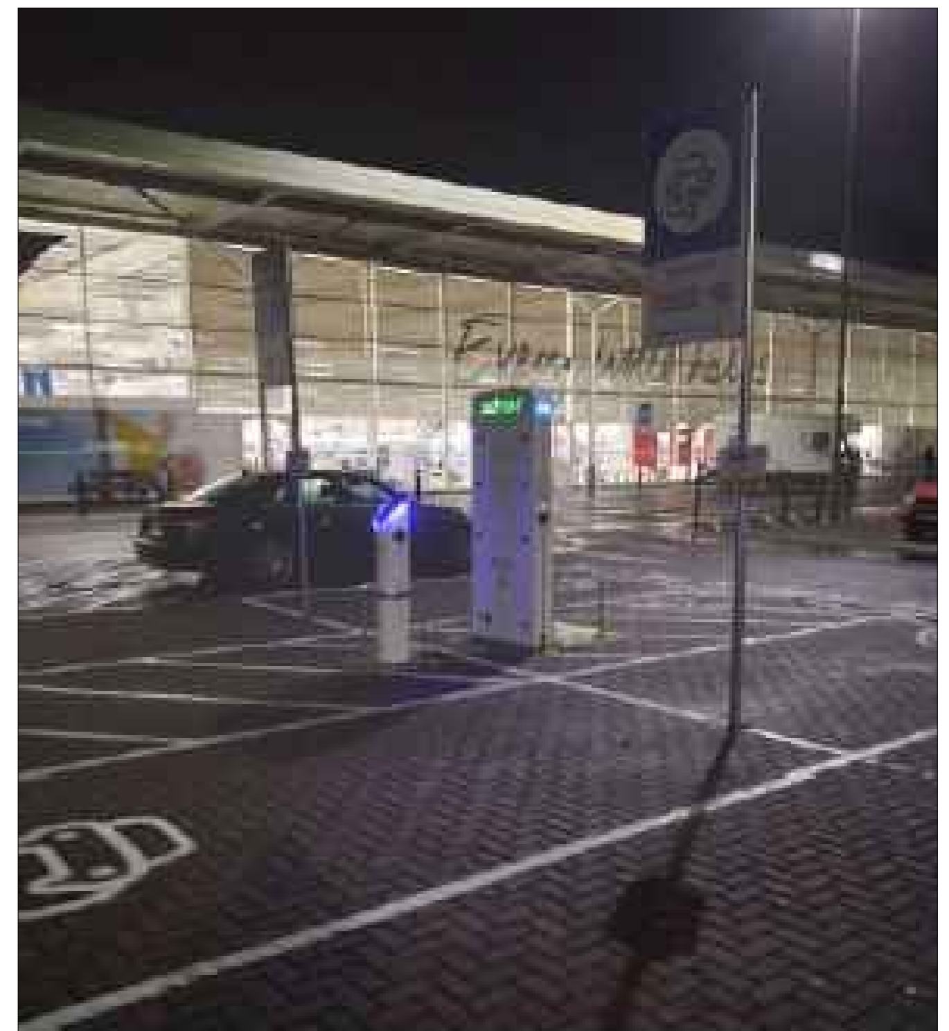
MEDIA CHARGER AND FAST CHARGER UNIT
