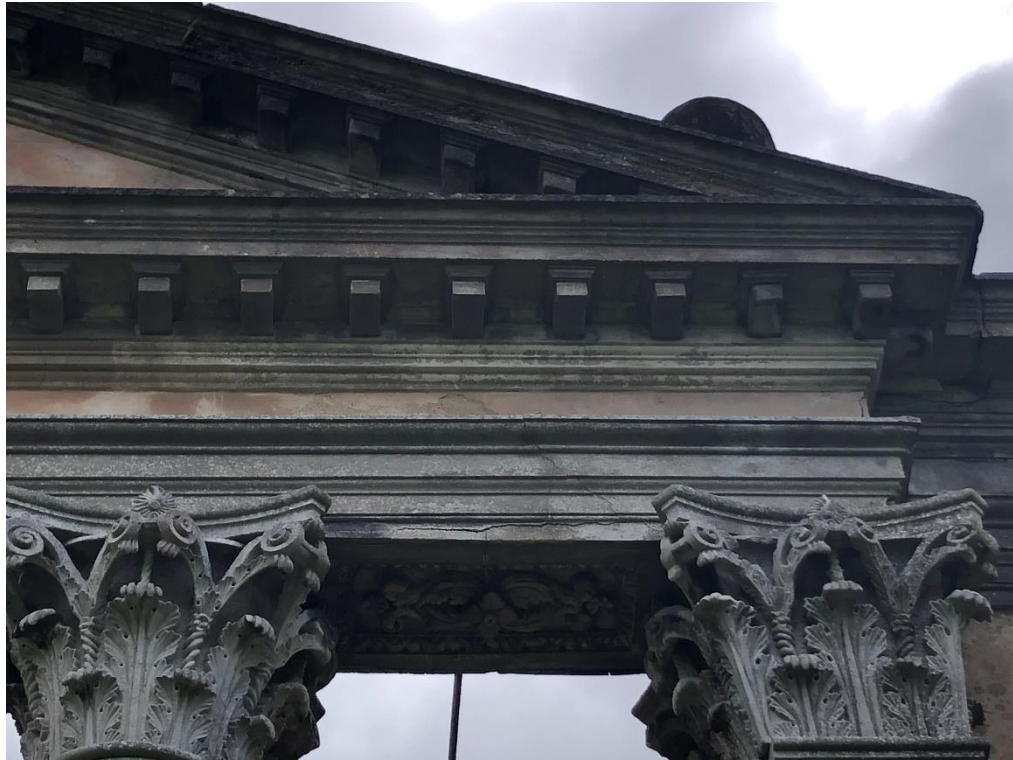
Adjacent cracking to render
