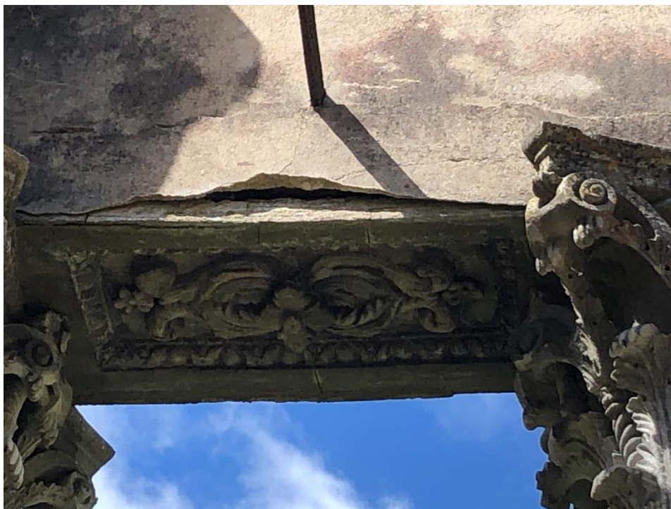
Cracking to base of internal render lining
