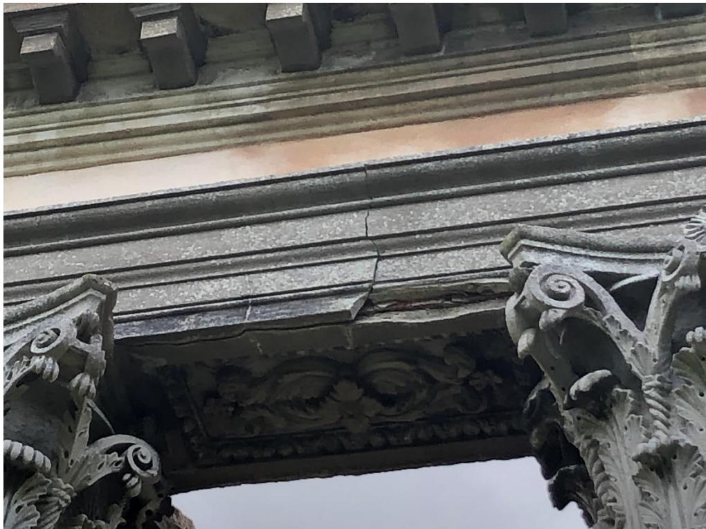
Fallen section of render, note cracking. Sound render above
