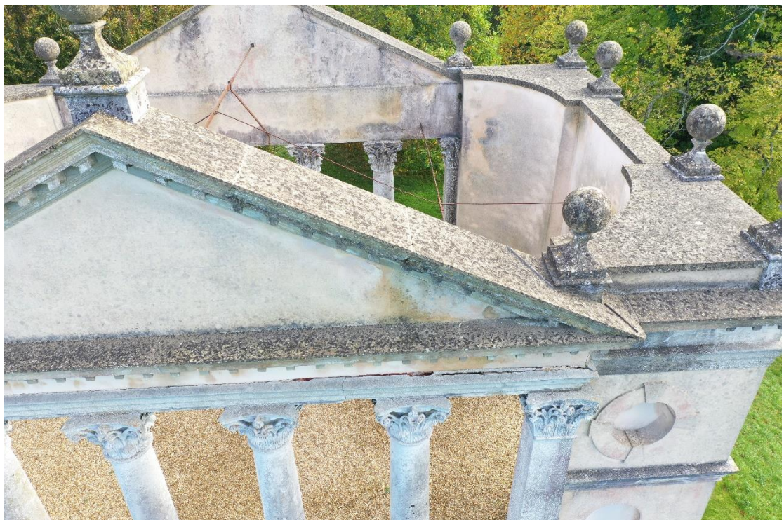
Significant crack to SW corner and destabilised string course
