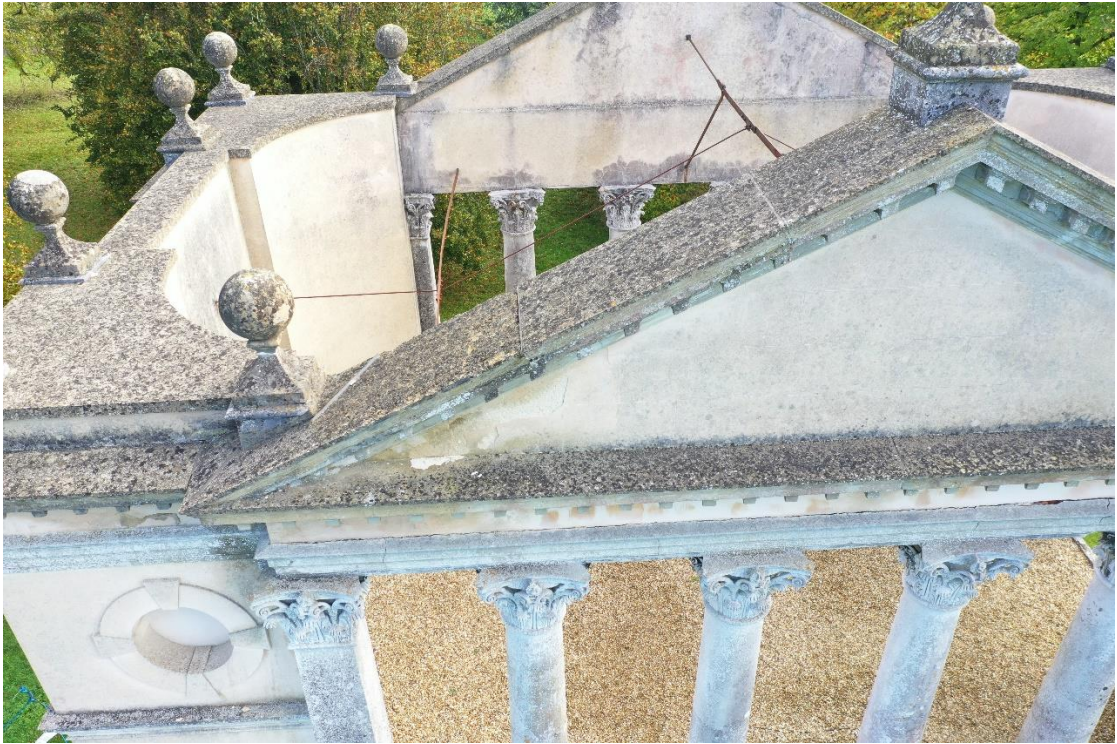
Finer crack to north-west end of west string course – full length
