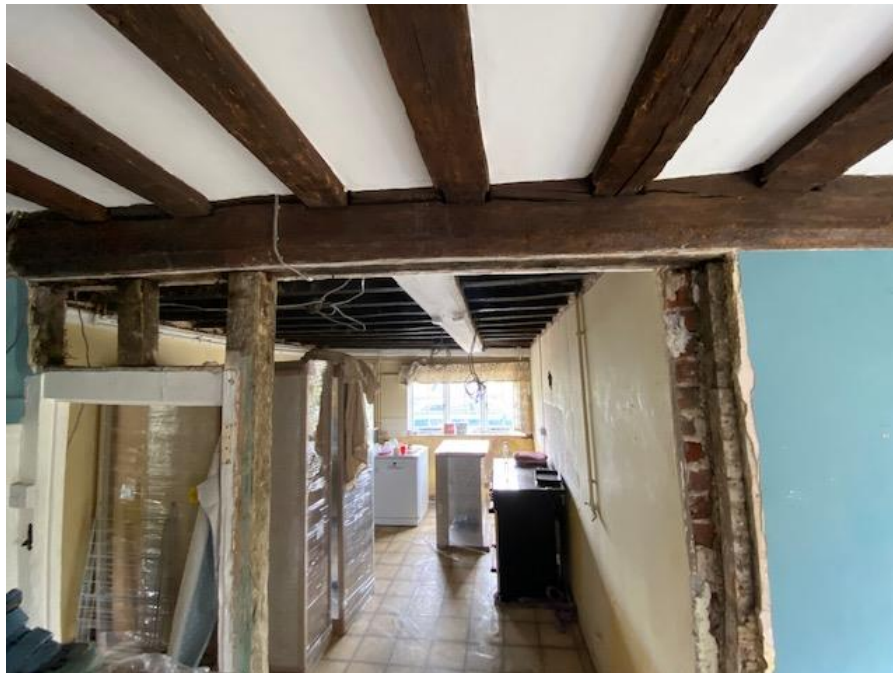
Picture 7. Location of Wall B in relation to the adjoining parallel running beam.
