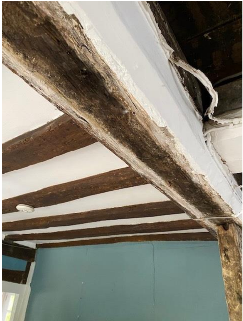
Picture 2. Beam above Wall A with no signs of mortice joints indicating that this wall was not original.
