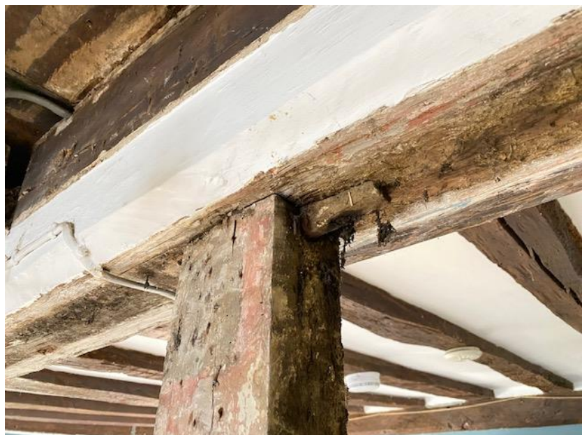
Picture 3. Studwork on Wall A is located and secured with nailed pegs onto the beam also indicating that this wall was not original.
