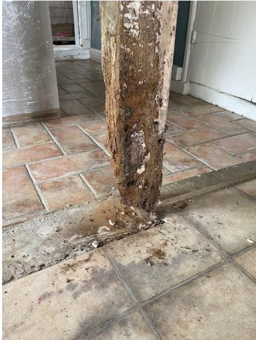
Picture 4. Timbers of Wall A showing significant deterioration.
