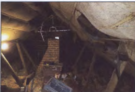
Figure 7: Loft space with tom felt to right of picture and cut of chimney in centre.
