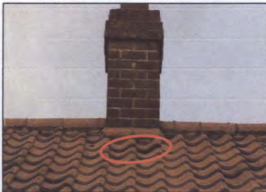
Figure 3: Close up of chimney with raised tiles at base.
