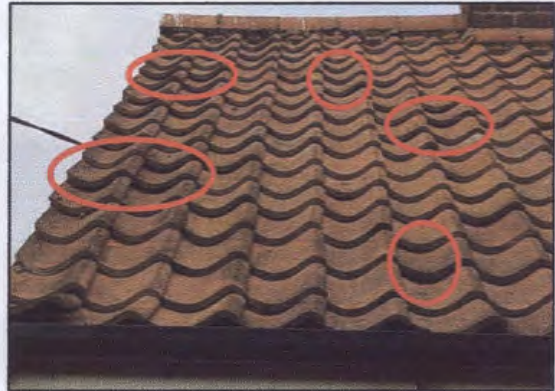
Figure 2: Close up of southern aspect roof at western corner, lifted tiles circled.
