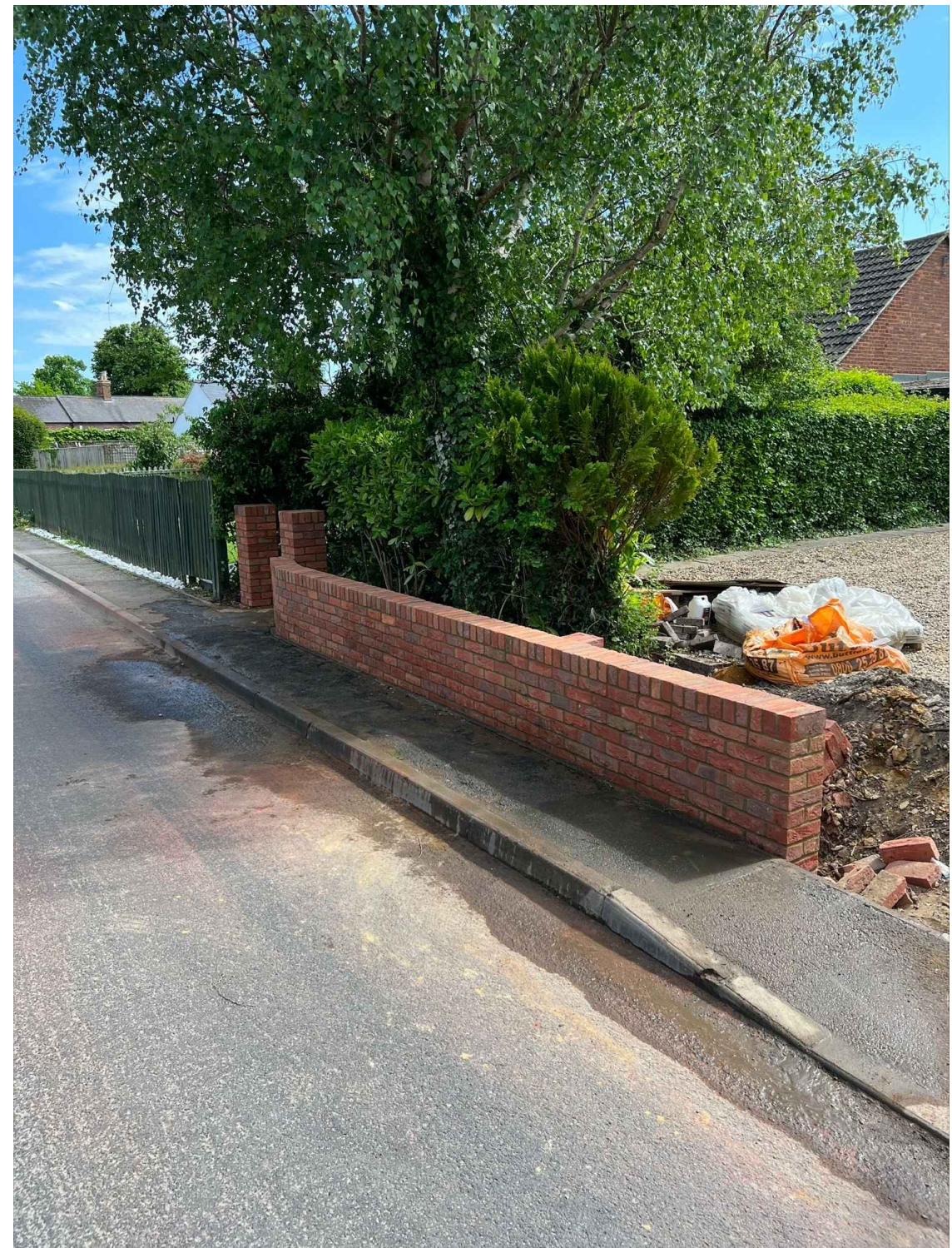
hedge removed & new brick wall built to back edge of footpath to a max 600mm high
