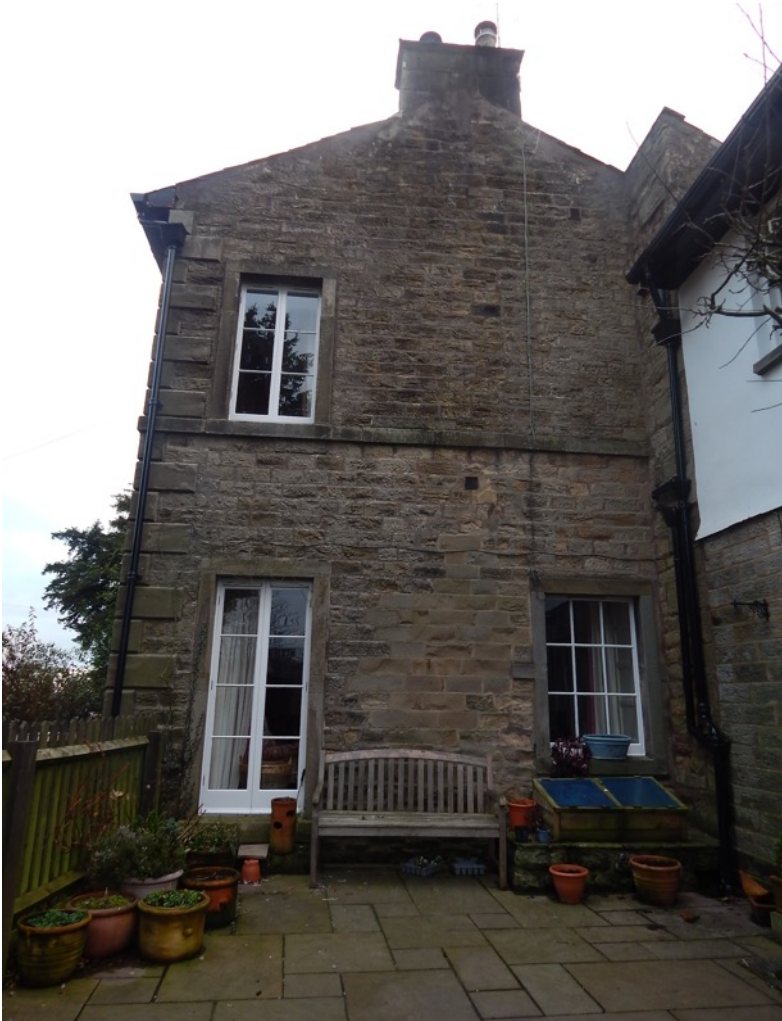
Figure 13 - Existing rear elevation – the view of the dwelling from the Church. Coal-hole in the foreground, right of centre
