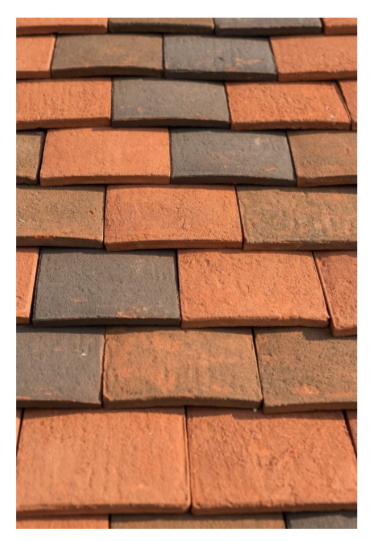
- Roof - Clay Plain Tiles (Orangery / Red) Black stained timber barge boards with plain tile undercloak Black stained timber fascia boards with exposed rafter feet Gutters and downpipes to be Roundstyle Cascade Cast Effect Gutter Heritage Black
