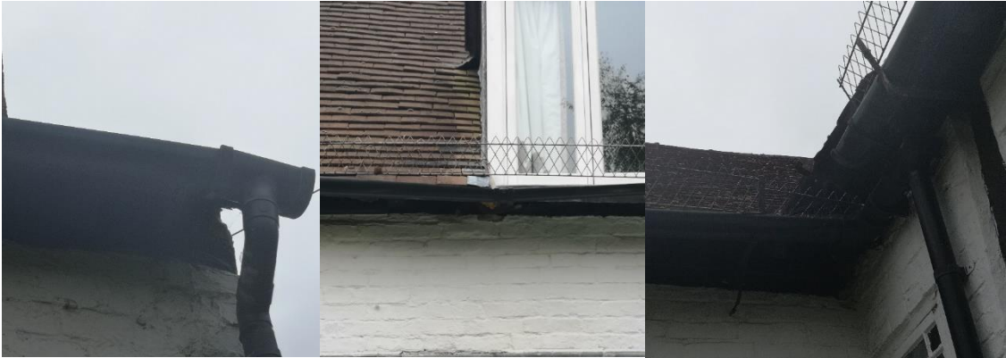
Examples of Worn out Rainwater Goods
