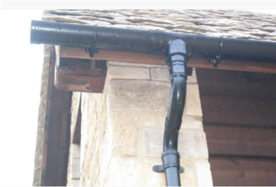
Gutters and Down pipes Black painted metal aluminium or cast iron
