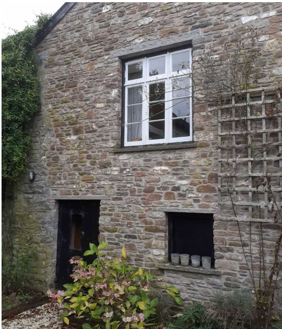
East gable of the barn, substantially re-built and a domestic style window inserted at first floor level.
