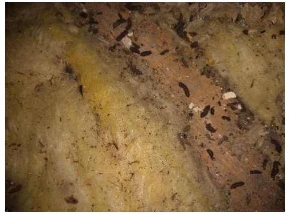
Photograph 6. Bat droppings found in loft space west of attic room
