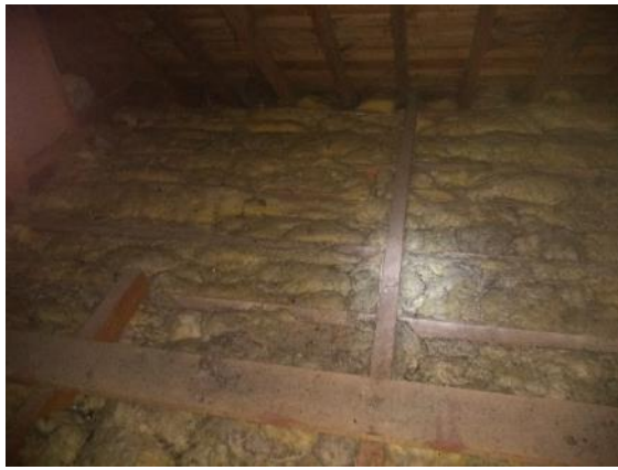
Photograph 5. Loft space west of attic room where roof space will be converted
