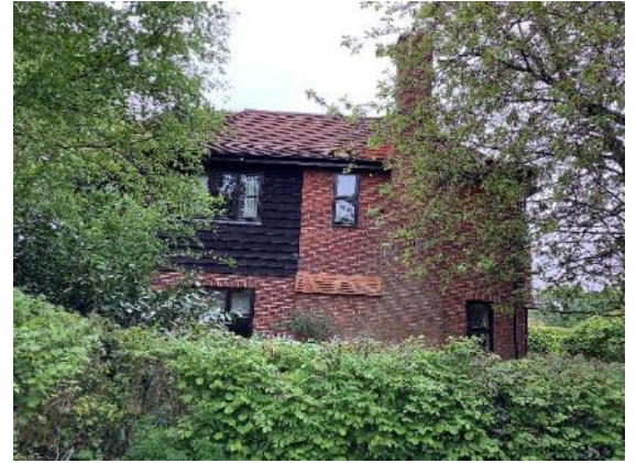
Photograph 2. West aspect of residential dwelling with gaps under hanging tiles, next to chimney, into the roof space
