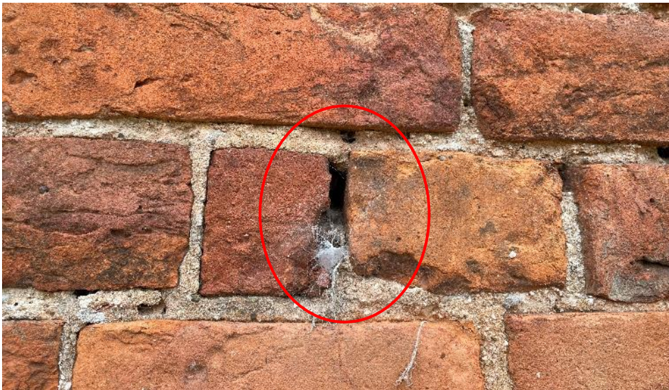
Example gap in the mortar between the brick-work (pictured above).
