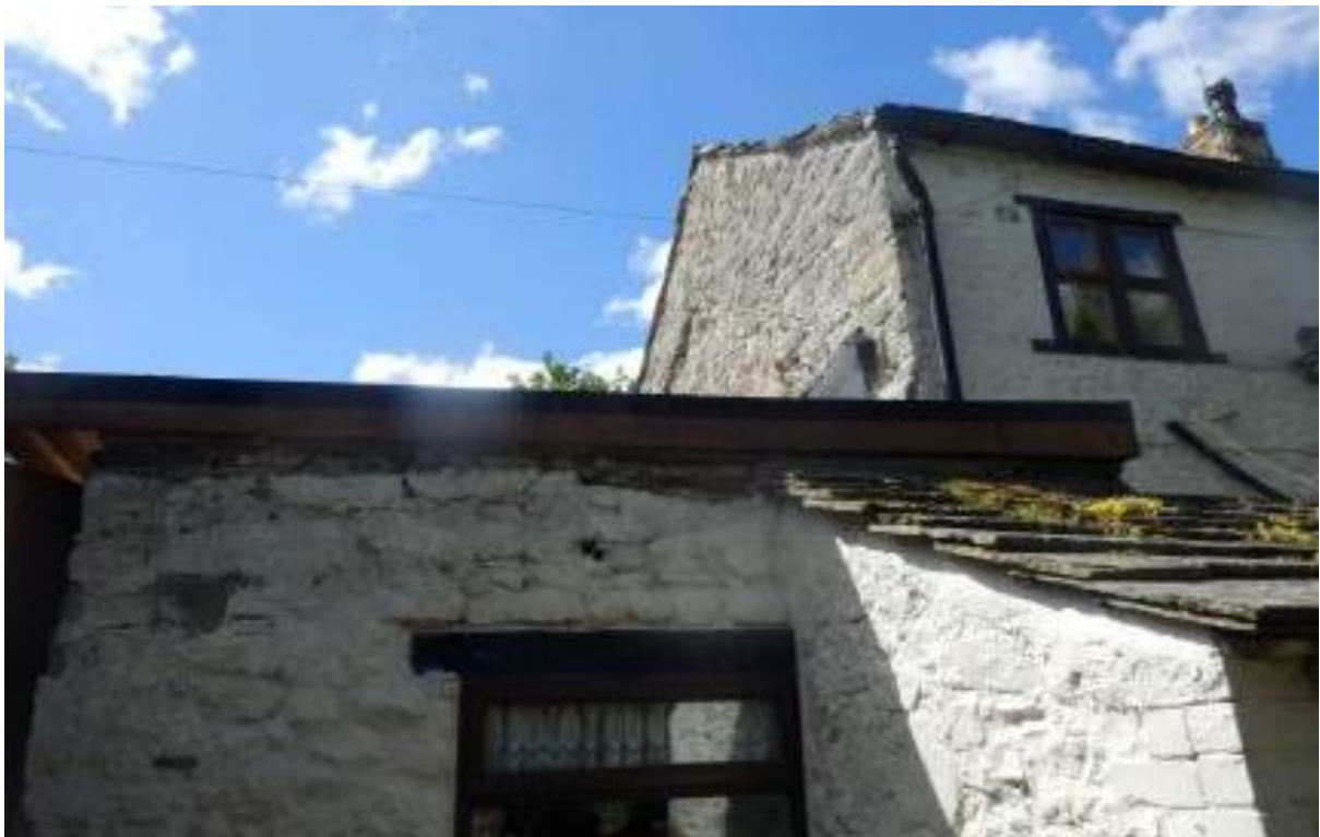
Image 4 Lean to and rear of the Dining Room with temporary roof over above.
