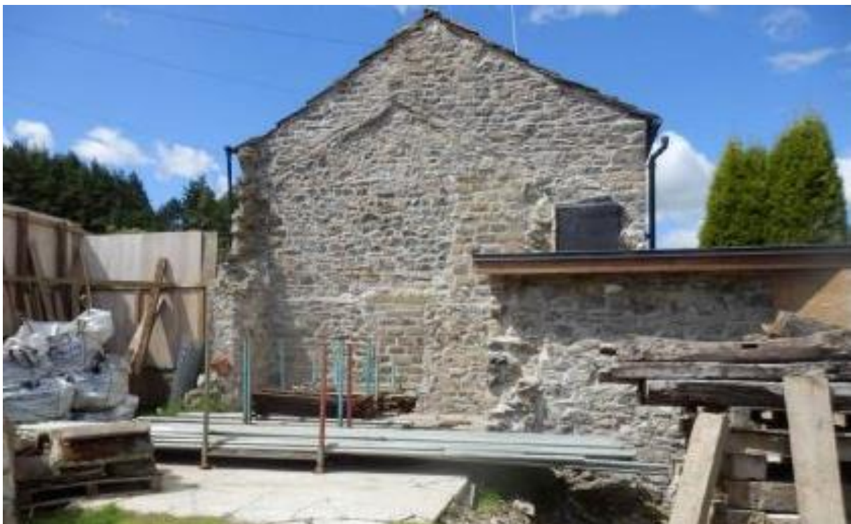
Image 2 Exposed party wall as at 21 June 2018. Dining Room to the property is in the single storey addition to the right of this photograph.
