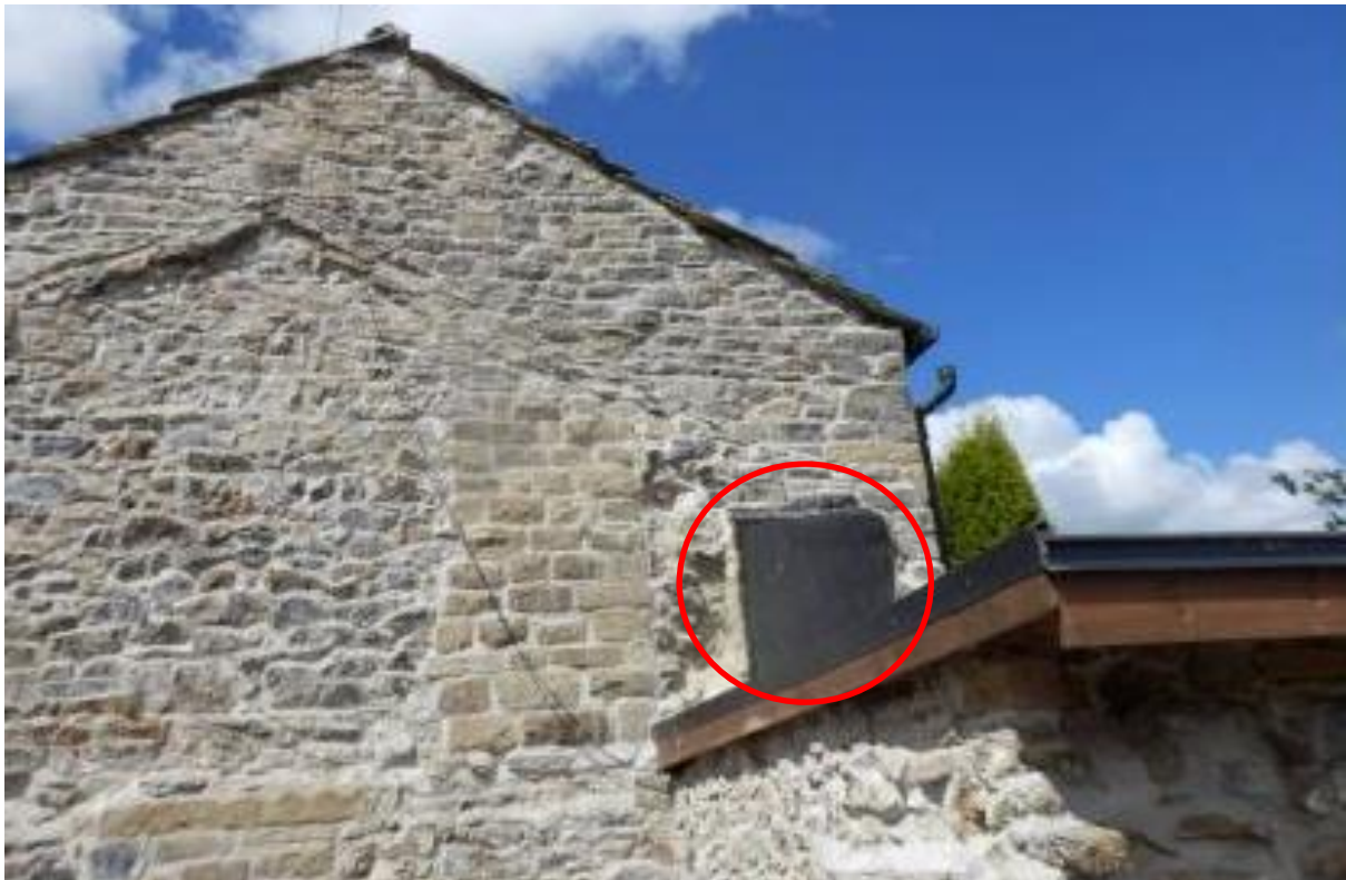
Image 3 View of infilled hole in the party wall when exposed following demolition of Nuttercote Farm.
