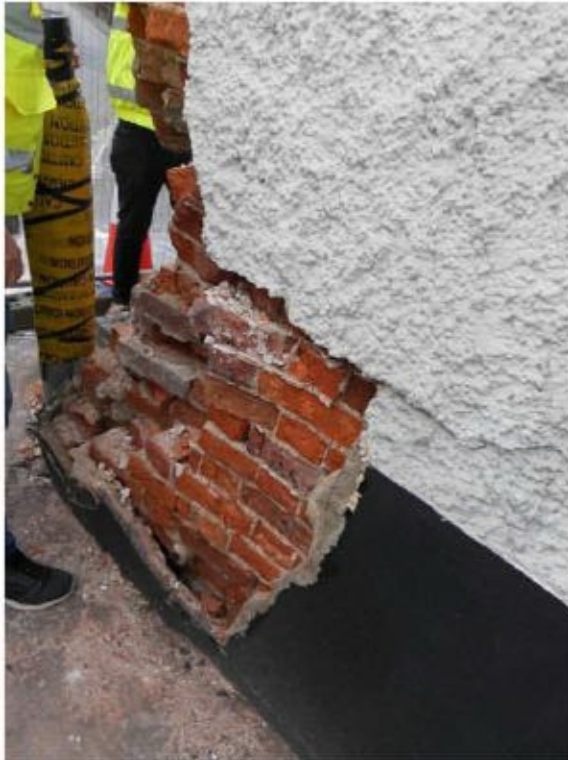
Impact damage to external wall. (Item 1 & 2).
