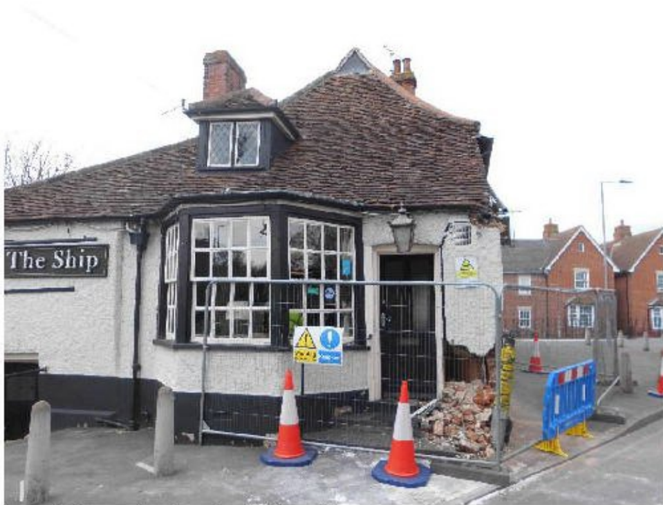
Impact damage to external wall. (Item 1).
