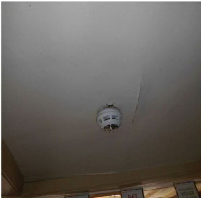
Sagging ceiling finishes. (Item 4).
