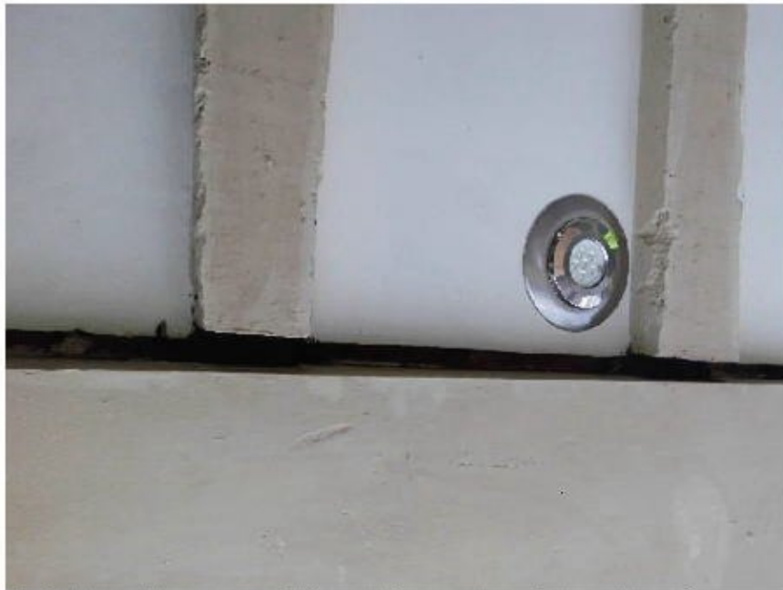
Partial loss of bearing to 1 st floor joists over bay window. (Item 3).
