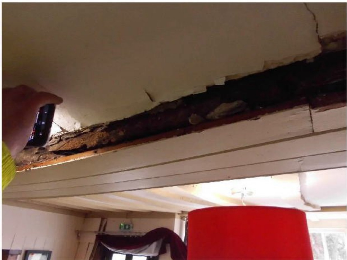
Excessively deflected Oak beam. Historic woodworm. Rot. Split beam. (Item 5).
