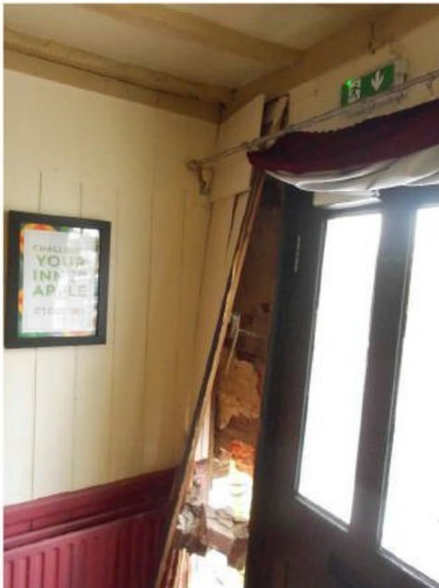
Impact damage to external wall, internal view. (Item 1).
