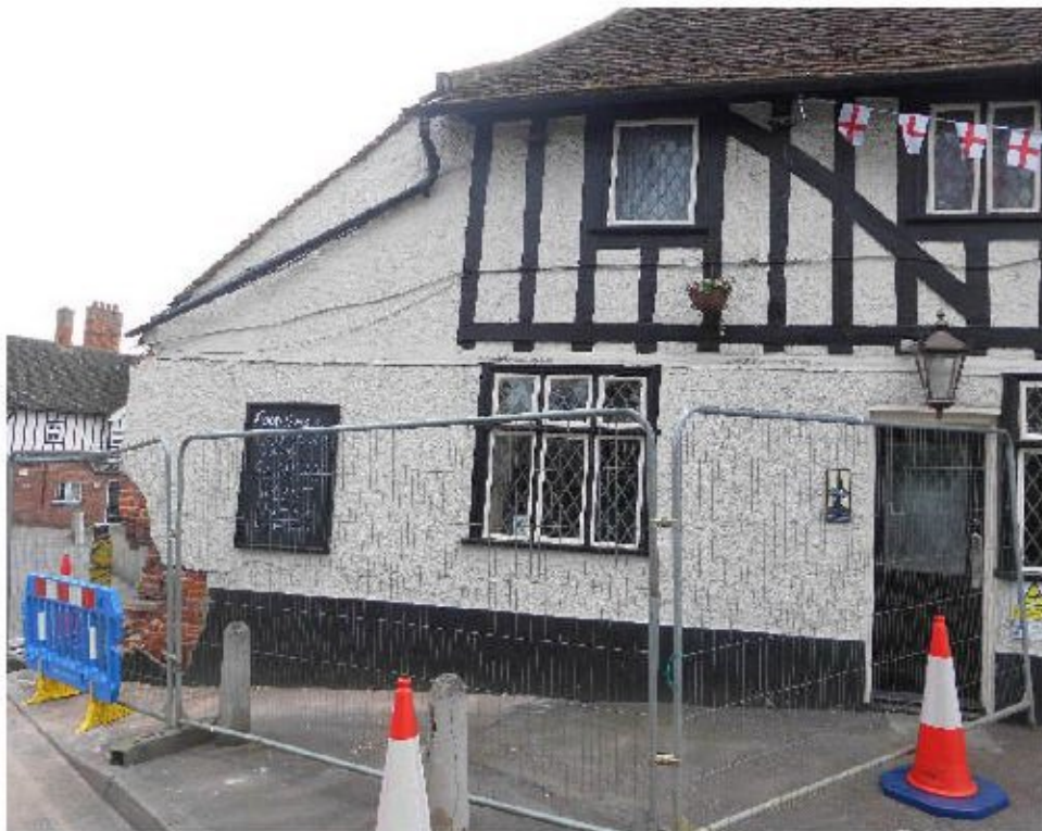
Impact damage to external wall. (Item 1 & 2).
