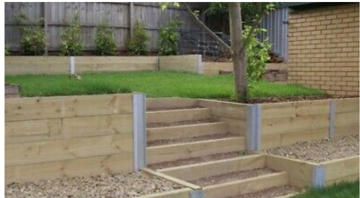
Wall Type 3 (W3): Rear Garden Embankment FSC Timber sleeper retaining walls, 600-1200mm high, forming 3 terraces (to Engineer's specification). Supplier: Contractor to propose local supplier
