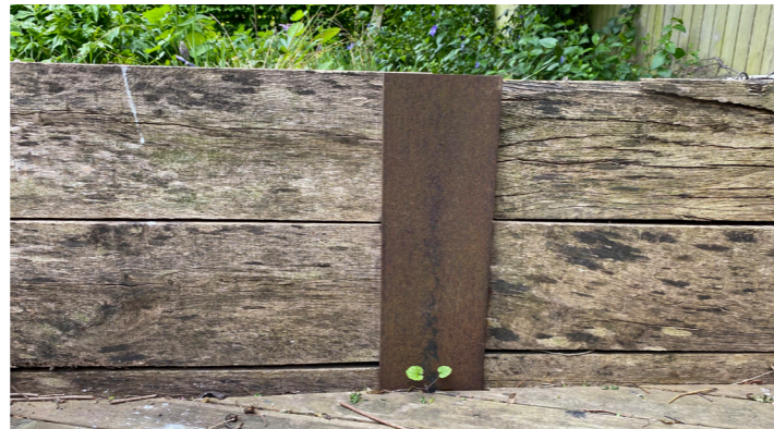
Wall Type 3 (W3): Rear Garden Embankment Timber sleepers are laid horizontally & supported by mild steel angle posts (to Engineer's specification). Supplier: Contractor to propose local supplier
