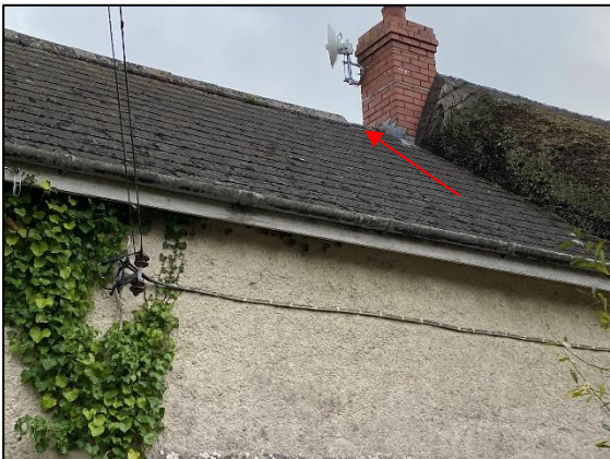
Plate 13: Missing ridge tile Lee Ecology
