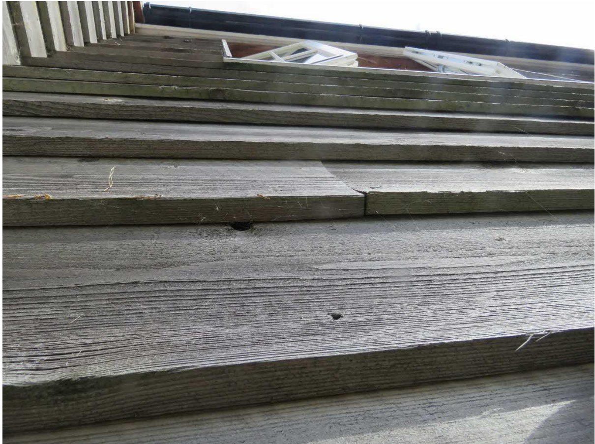
Figure 4. Showing close up of tightly fitted wooden cladding and small, cobwebbed knot-hole.
