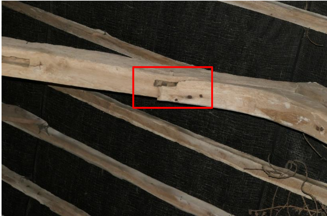
Photo 1 , mortise and tenon joint with common pipistrelle, highlighted in red, located within the main barn on the 1 st December 2021 and 4 th January 2022.
