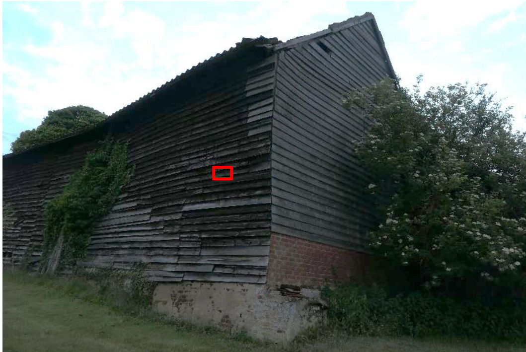
Photo 6 , common pipistrelle exiting the barn via weather boarding on the west, highlighted in red. 4 th May 2022.
