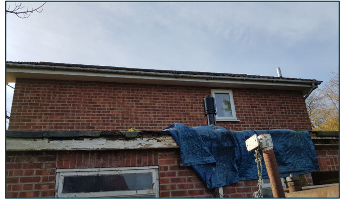
Hole in flat roof (side)
