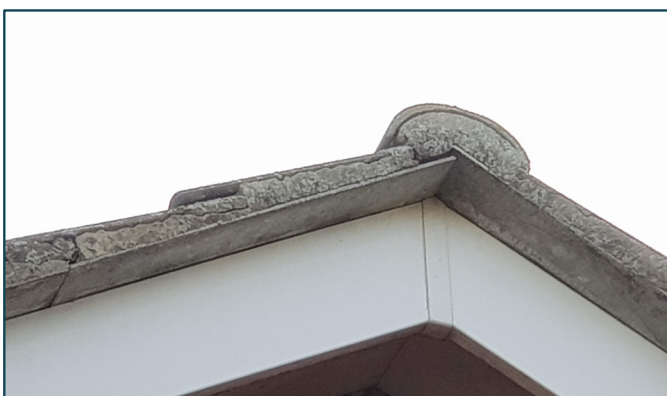
Missing mortar at rake
