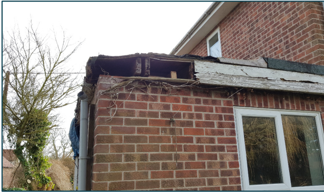
Hole in flat roof (rear)
