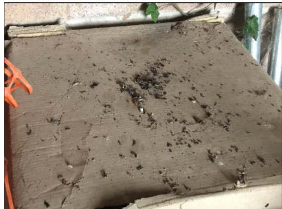
Photo 2: Clustered bat droppings amongst debris
