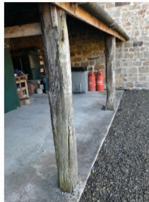
EXISTING TRACTOR LODGE HAS A CONCRETE FLOOR ON A PLASTIC DPM. STONEMWORK SHOWS STRUCTURAL CRACKS TO BACK WALL. ROOF BOWING AND SHOWING CORROSION TO METAL CORRUGATED SHEET. TIMBER COLUMNS CRACKED AND WITH EVIDENCE OF ROTTING AT GROUND LEVEL.
