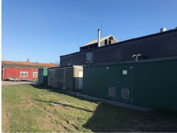
Figure 4: Existing substation at Manor Farm
