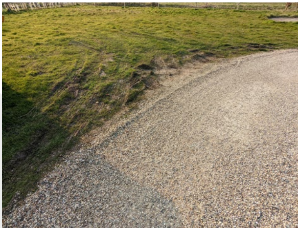
Photograph shows the damage to the grass at the corner of the drive, caused by delivery vehicles using this as a turning point.
