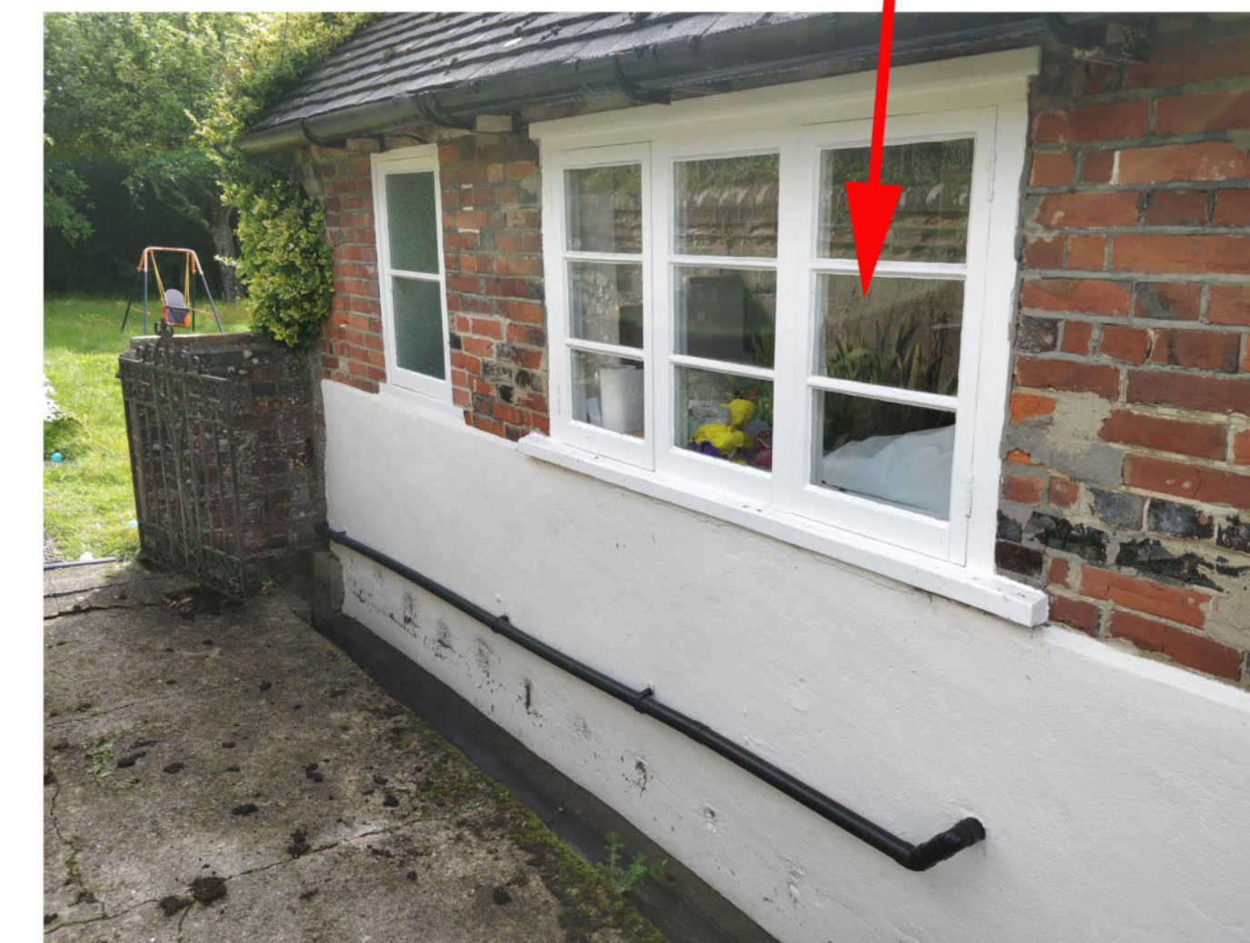
Existing Window to be replaced with door and window
