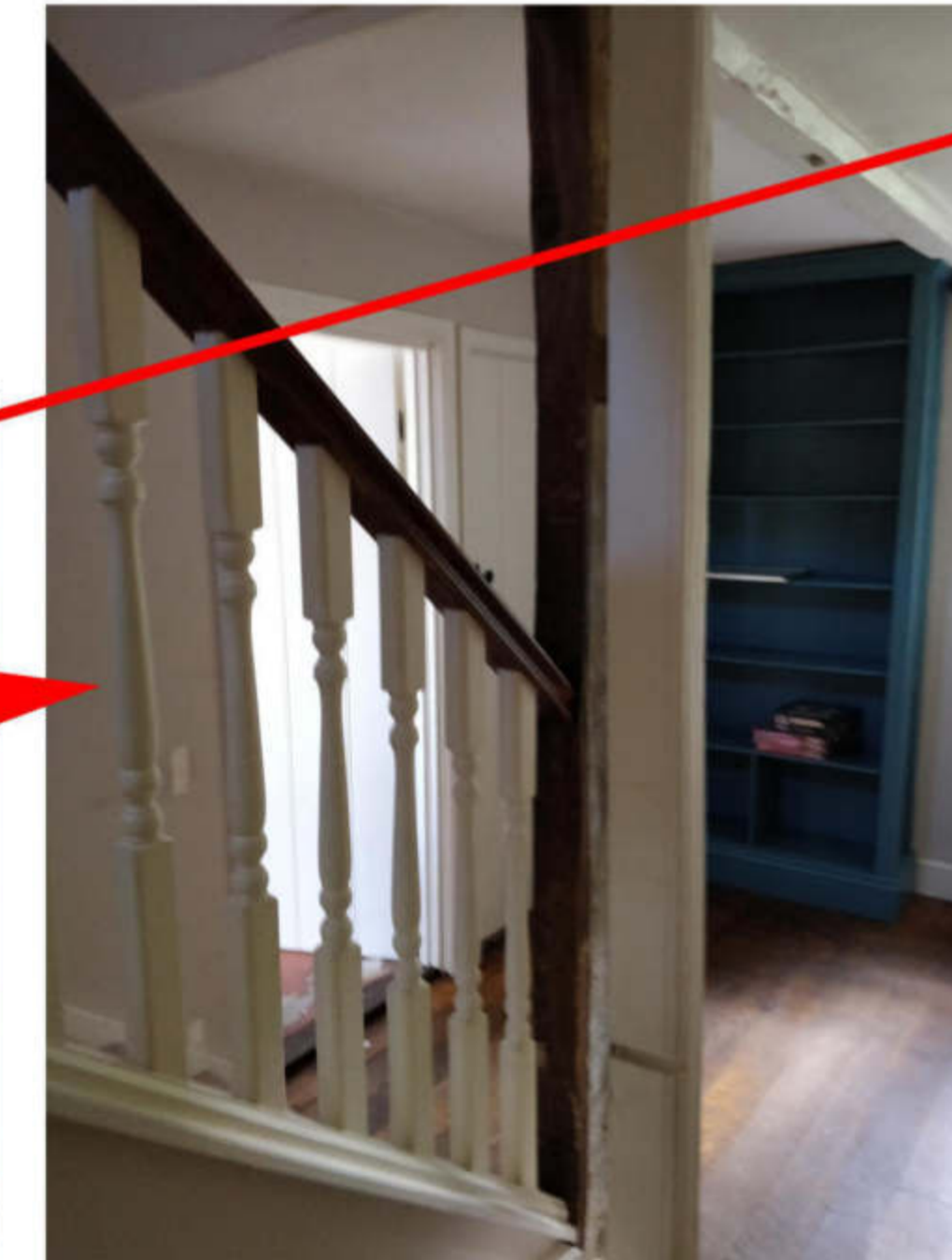
Existing Baluster (To be removed)
