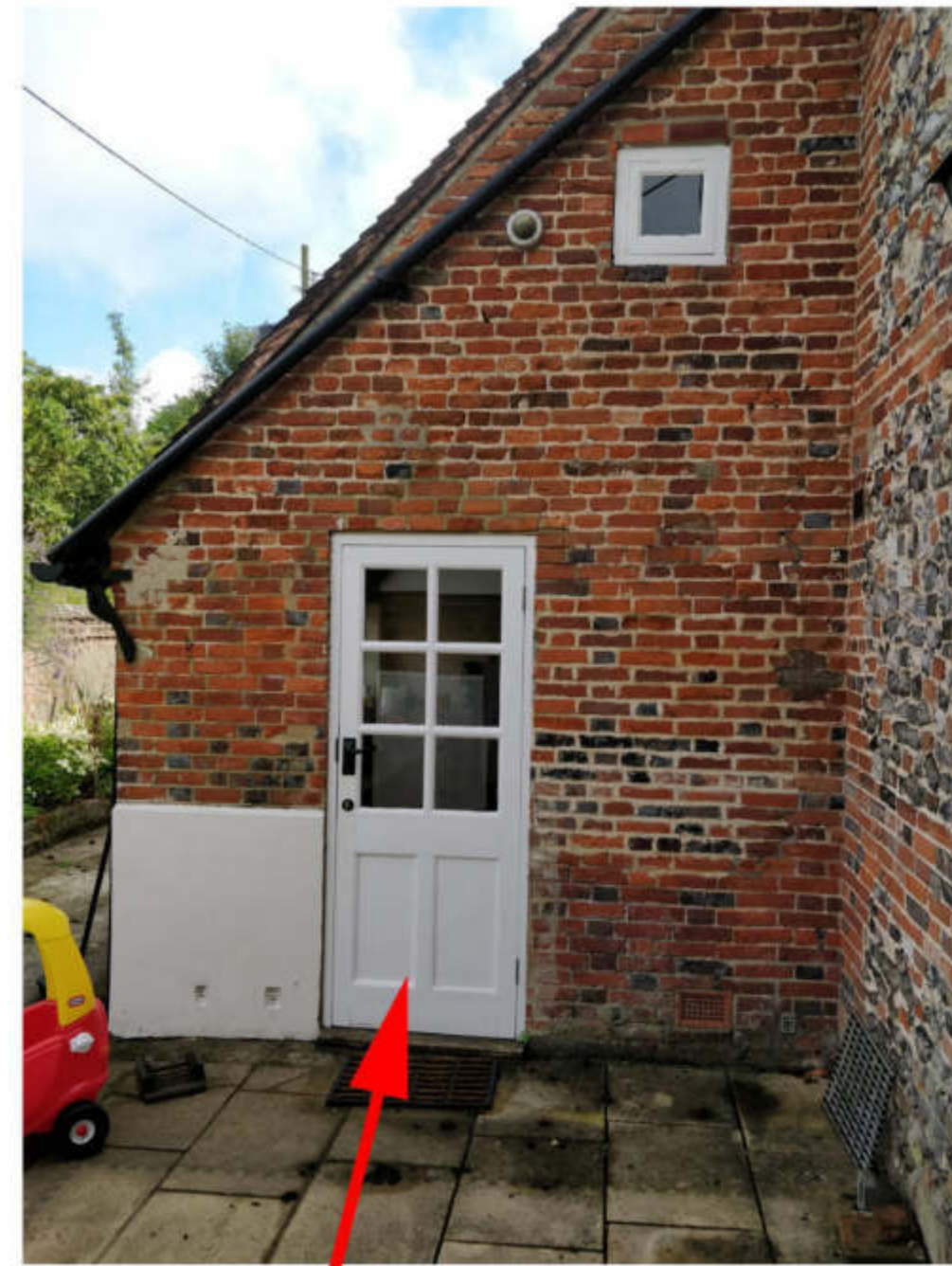
Existing door to be infilled (Leaving recess)
