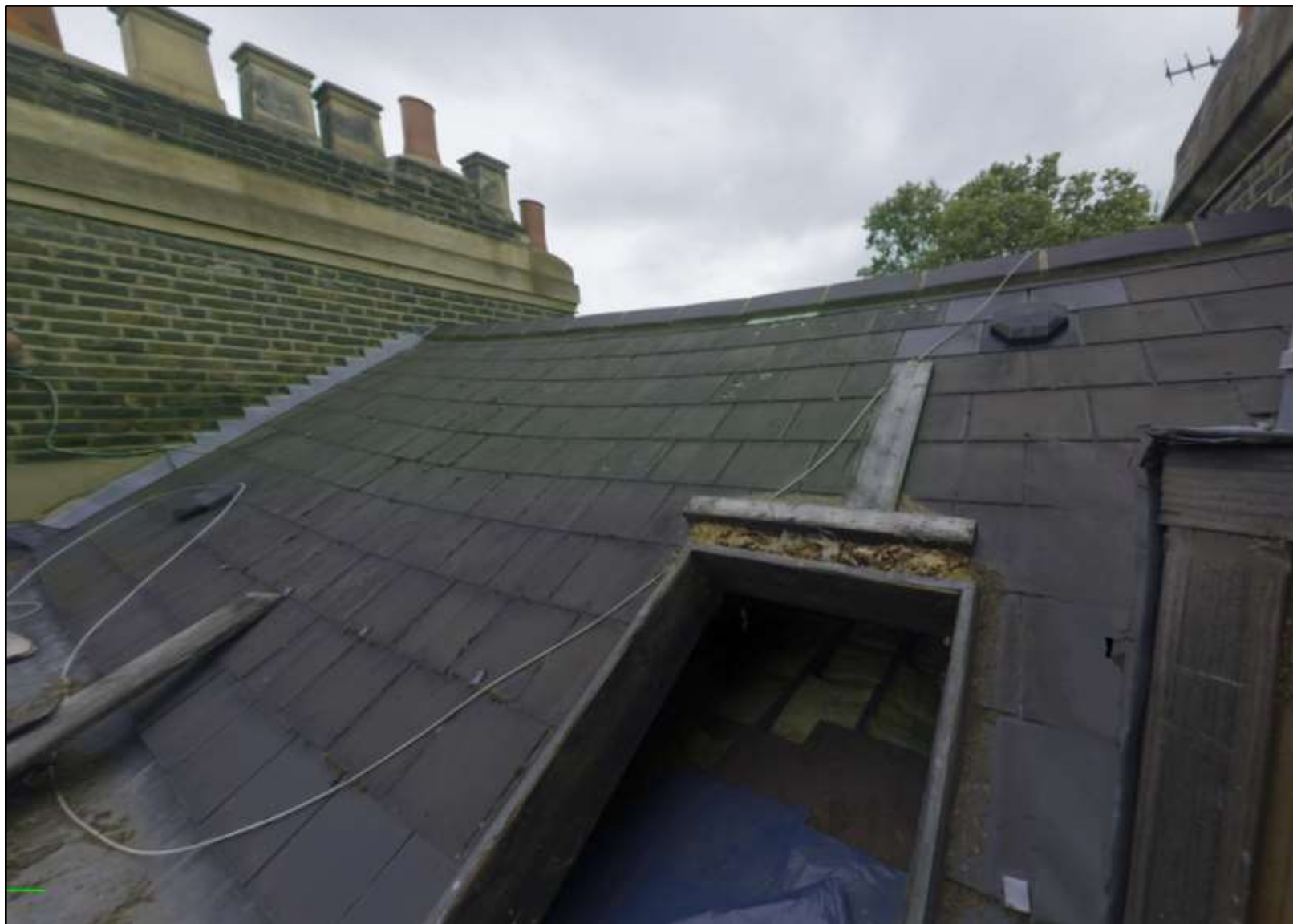
Figure 21: External view of the roof- the repairs to the lead flashing and new ridge tiles are evident
