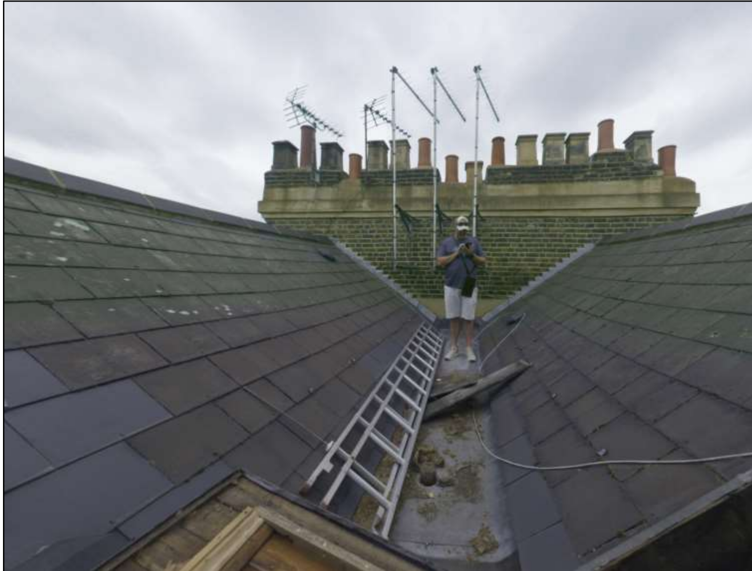
Figure 20: External view of the roof. Note the patch repairs with new shingles, ridge tiles, and lead flashing. Also note the gully that runs through the centre of the roof parallel to Belgrave Road.
