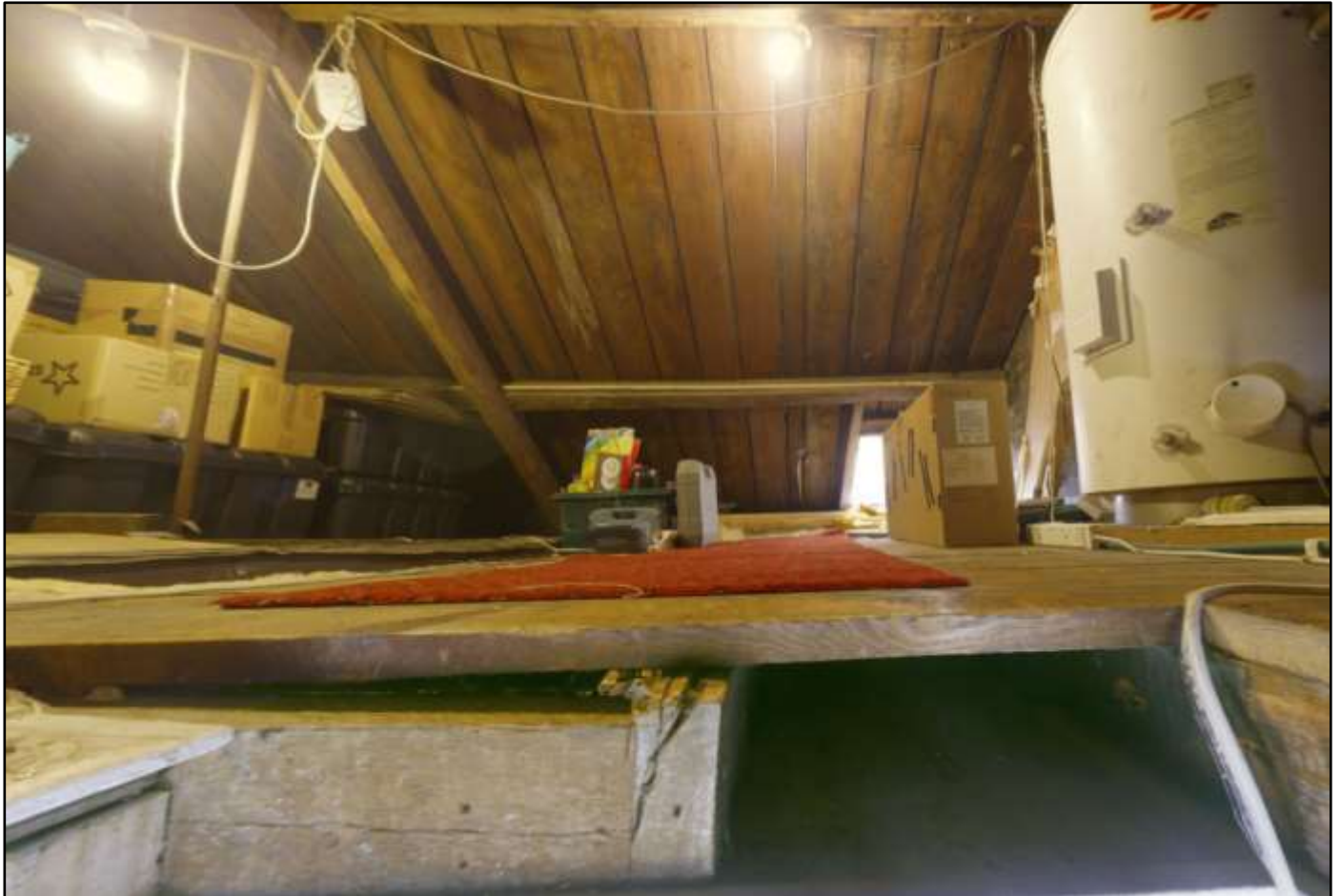
Figure 17: View of the attic space when viewed from the hatch leading from the kitchen. Note that a floor has been laid and insulated in part.
