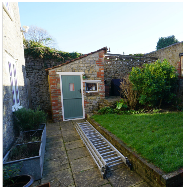
Fig. 3. View of the existing outbuilding built without permission by a previous owner with its leaky roof and narrow door making it too small to usefully store bicycles or other household/garden items.
