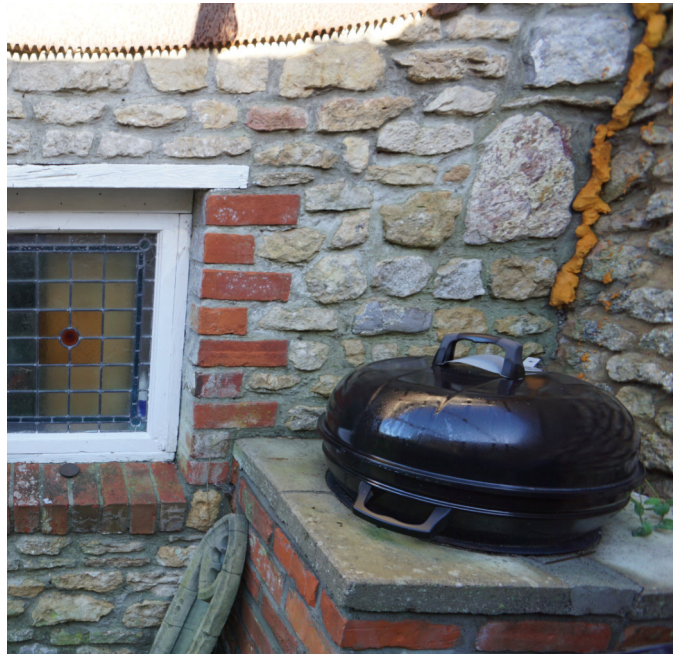
Fig. 5 Existing outbuilding pulling away from the neighbouring wall (built without proper ties) resulting in cracks and leaks throughout the structure. Expanding builders foam used to RHS by previous owner in an attempt to achieve waterproofing.
